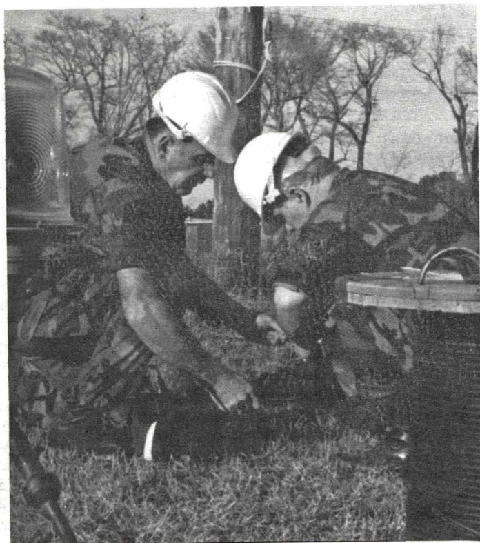
SMSgt. James Devitt and MSgt. Paul Bates check the wiring as they prepare to light up the airfield.
