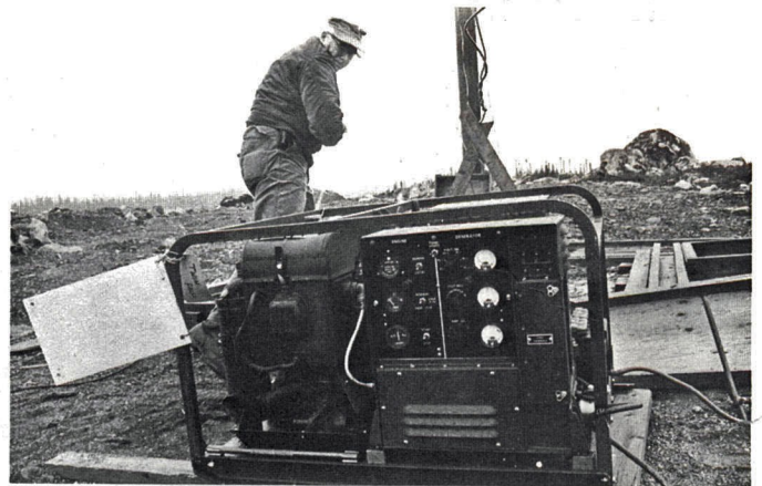
MSgt. Arthur Needham tugs on a generator starter cord. Generator power was the sole source of electricity at Twin Falls.
