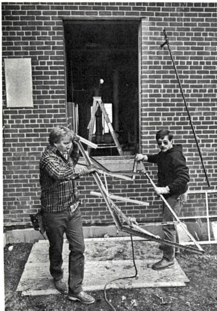
Roland Ohsborne (left) and Ken Doucette pull out old, drafty windows at the Reserve Recruiting building. (USAF photo by Capt. Philip Weber)
