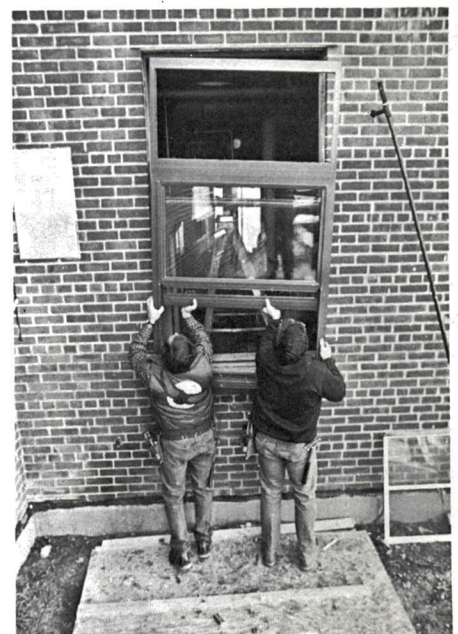
Joe Petrone (left) and Ken Doucette install new energy efficient windows. (USAF photo by Capt. Philip Weber)
