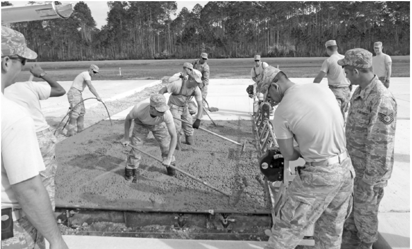
CONCRETE TRAINING >> Reservists with the 439 th Civil Engineering Squadron work wet concrete for a patch in this simulated "bombed" runway. This was part of CE's Prime Beef training held at Tyndall AFB, Fla., in January. For the story and photo, visit Westover's web site at westover.afrc.af.mil. (photo by TSgt. Eric Tupaj)
