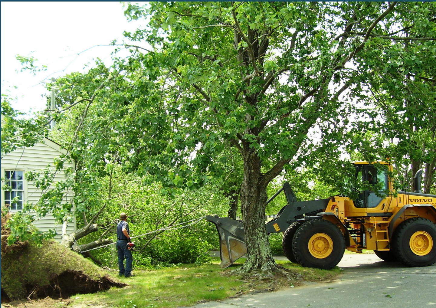
STORM DAMAGE >> A repair crew cleans up damage from a May 26 storm which knocked a tree over near the base chapel section of Bldg. 1100. Dan VanDalsen, real property maintenance manager with Phoenix Management Inc. at Westover, took this photo of the storm's aftermath. Photographers are encouraged to shoot high-resolution photos of Westover happenings and people for this back page photo section of the Patriot . Photos may be submitted to 439aw.pa@westover.af.mil.
