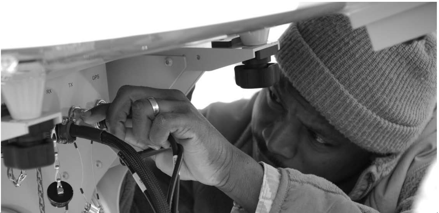
PLUGGING IN >> Tech. Sgt. Desmond Farrell, 439th Communications Squadron works on the Joint Incident Site Communications Capability system in April. (photo by Senior Airman Andre Bowser)
