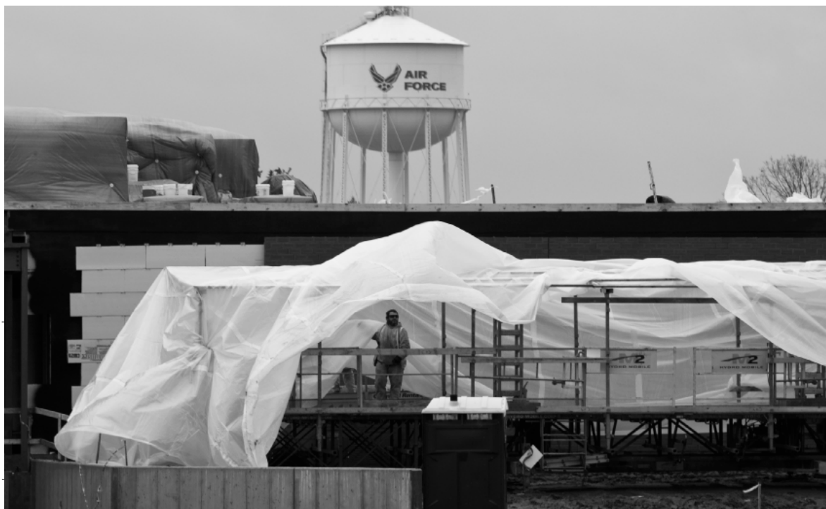
BUILDING A JOINT FORCE >> Construction continues on the Armed Forces Reserve Center, a 75,000-square foot building quickly rising across the street from the military personnel flight. By the fall, about 1,000 Army soldiers will occupy the building. (photo by Master Sgt. W.C. Pope)
