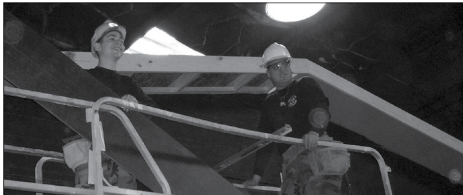
NEW HOME >> Airman 1st Class Anthony Tassinary (left) and Senior Airman Greg Paczkowski install trim on a modular home built for Native Americans. ( photo by Senior Master Sgt. Michael Herens )
