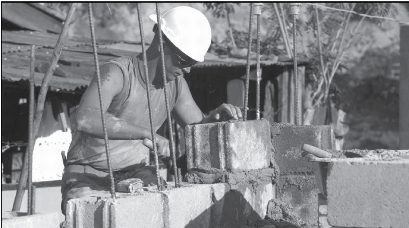
THE BEDROCK OF A GOOD EDUCATION >> Marine Cpl. Ross Jupert, a member of Westover's Marine Wing Support Squadron 472nd Detachment B lays block at the Gonzolo River school construction site in La Ceiba, Honduras, as part of Operation New Horizons 2006. (photo by Tech. Sgt. Maria Bare)
