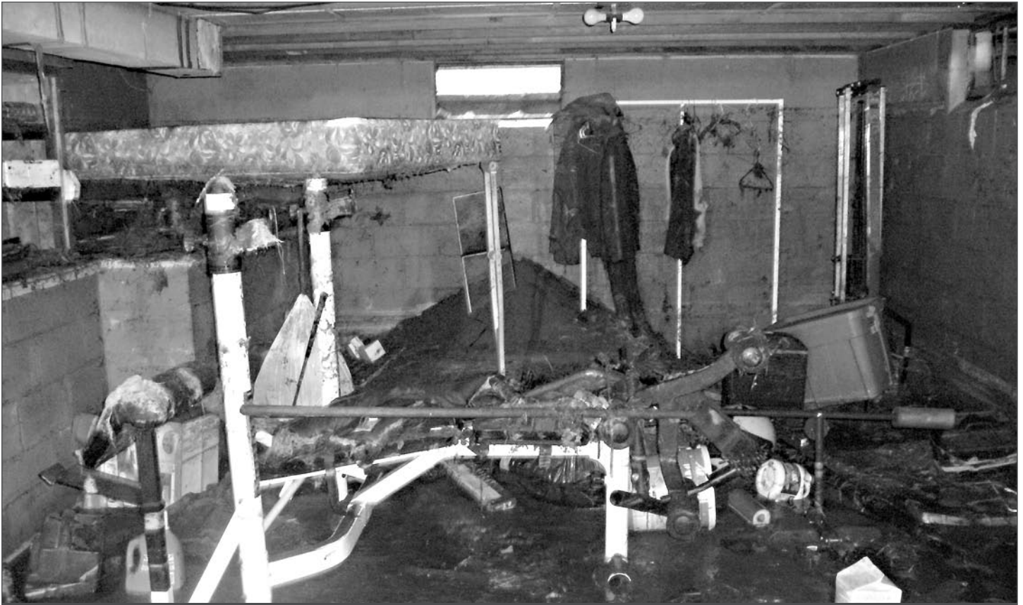
TOTALED >> The basement of Senior Master Sgt. Ann Fluegge lies in destruction after a nearby beaver dam collapsed, flooding the surrounding area.
