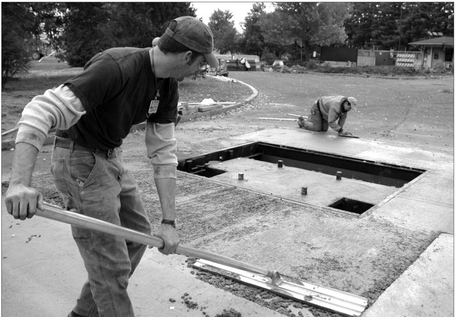
SMOOTH SURFACING >> Clayton Gray, with Secure Applications Inc., smooths out concrete over one of the pop-up barriers at the James Street Gate. The barriers are part of new security measures taken to protect Westover. Crews have installed the barriers at the new Westover Road gate as well.
