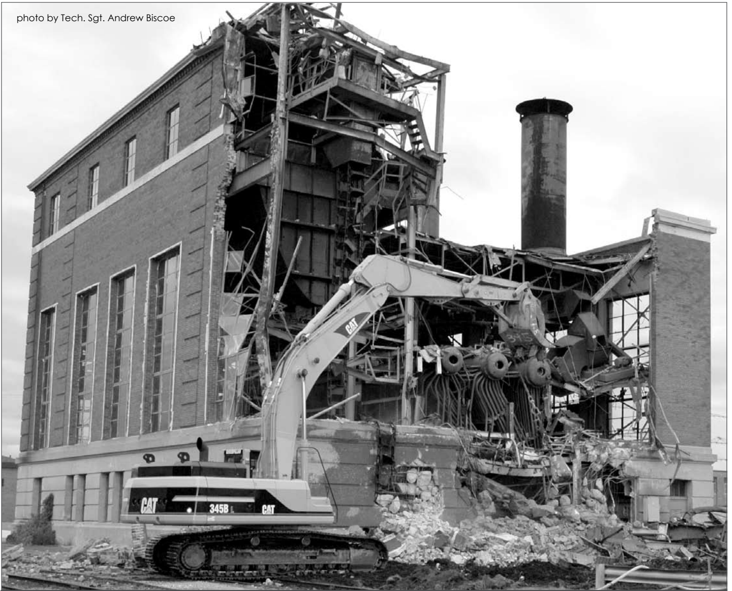
DEMOLITION DAY >> An excavator operator uses a wrecking ball to demolish Bldg. 1411, the former central heat plant, Oct. 27. The heat plant, located on Hangar Avenue, was built in 1940 and provided heat for all Westover buildings until 2003, when the base went to a decentralized heating program. Each building now has its own heat system. Ninety-five percent of the building's materials - including steel, brick, and concrete - were to be recycled, said Leroy Clink, base civil engineer. The demolition took about two weeks.
