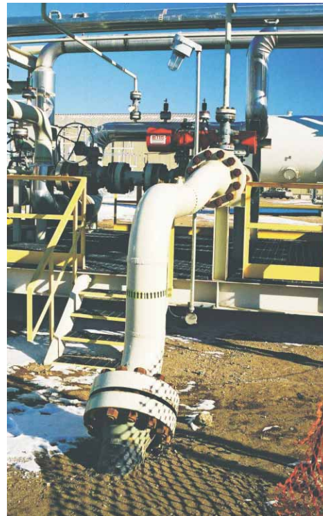
Pipeline carrying CO 2 from North Dakota, USA, emerges from the ground at Weyburn, Canada.
