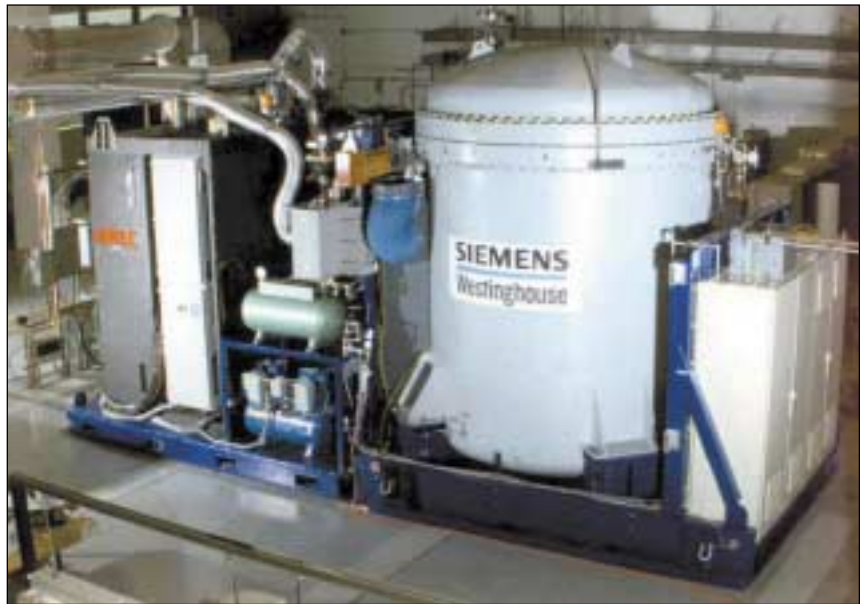
Siemens Westinghouse fuel cell/turbine hybrid system
