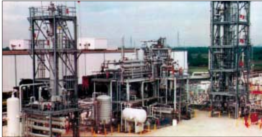
Air Product's LaPorte coal liquefaction test facility contributes to R&D efforts that ensure future availability of clean, affordable coal-derived fuels.
