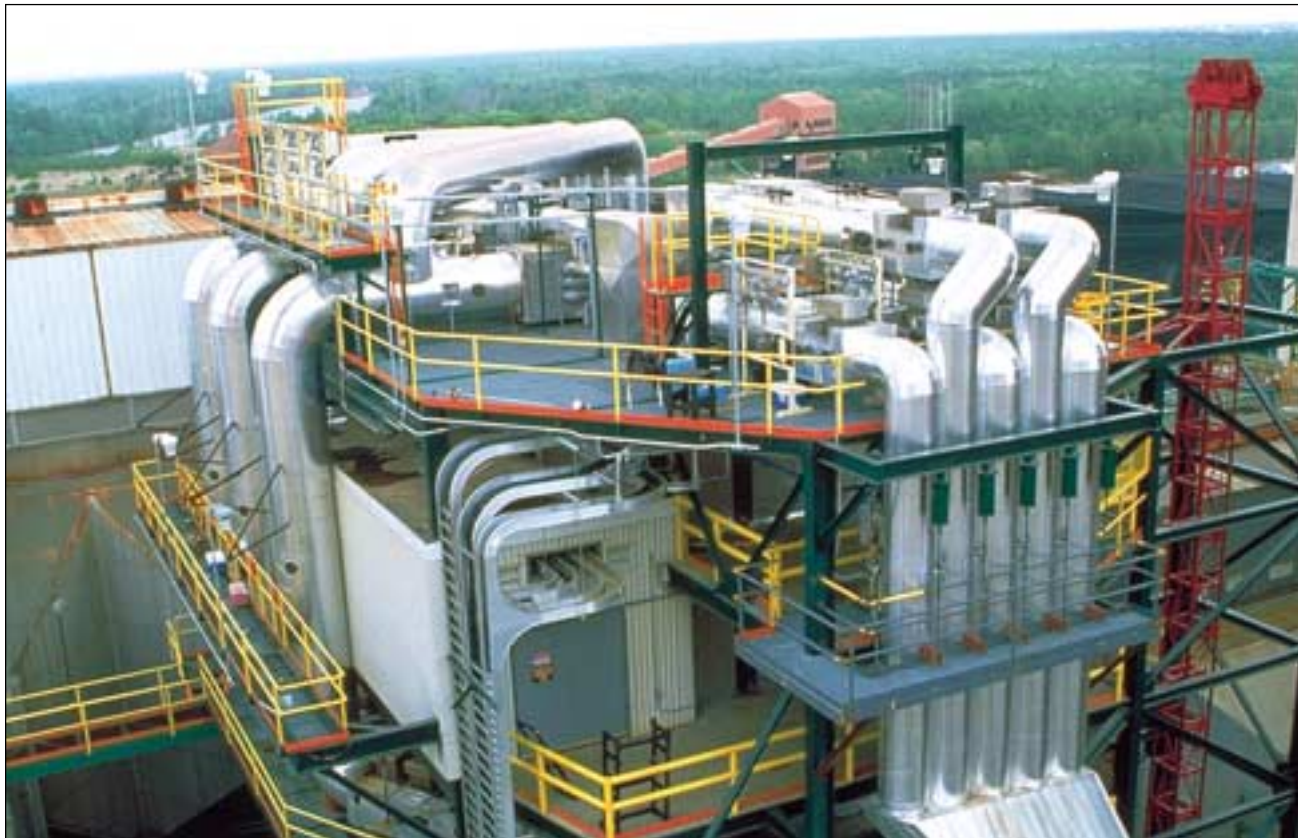
SCR test facility at Gulf Power Company's Plant Crist
