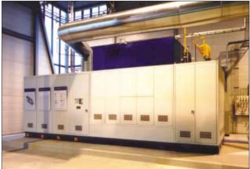
100-kW SOFC cogeneration system operating in the Netherlands, built by Siemens Westinghouse
