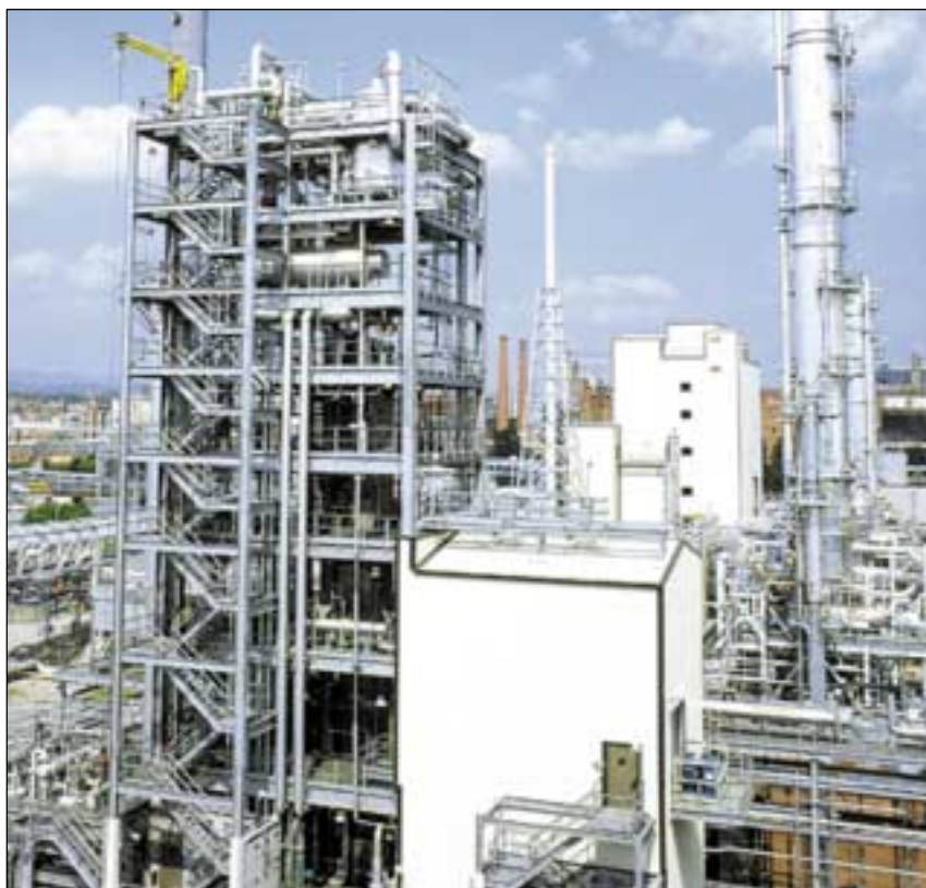
LPMEOH™ 80,000 gallon-per-day demonstration unit at Eastman Chemical Company's Kingsport, Tennessee Facility
