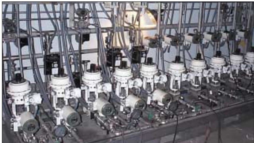
Metering pumps for the Cardinal Plant SNCR system's urea injection
