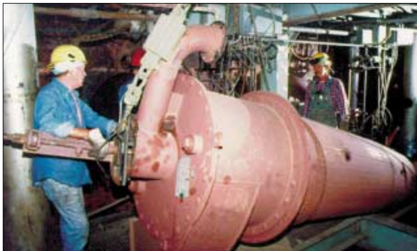
Low NO x burner installation at Gulf Power Company's Plant Hammond, Coosa, Georgia
