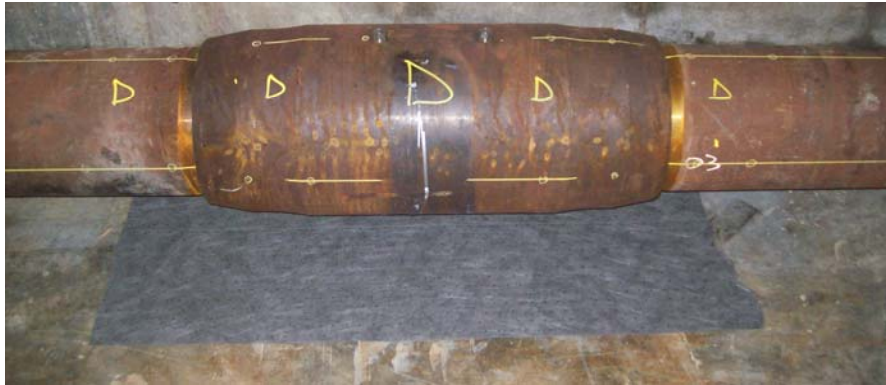
Absorbent Pad Under Coupling To Monitor for Leaks
