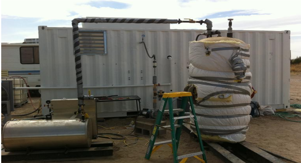
Figure 36: Field prototype near the wellhead. The prototype in its trailer is located in the background, and the water pre-heating system for this configuration is shown in the foreground, including a small insulated tank and a steam generator.
