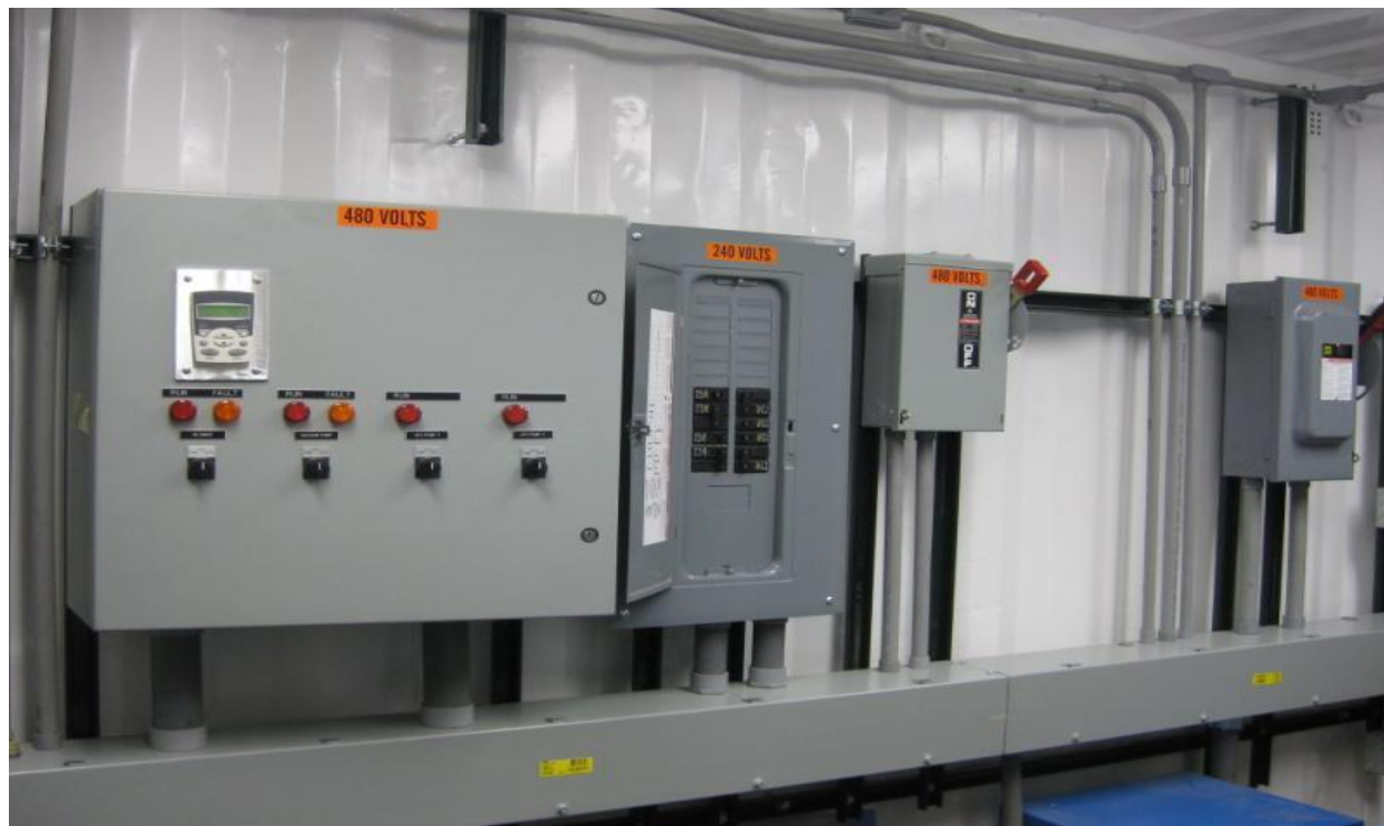
Figure 30: Electrical controls for the unit.
