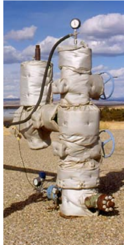
Insulated CO 2 source wellhead
