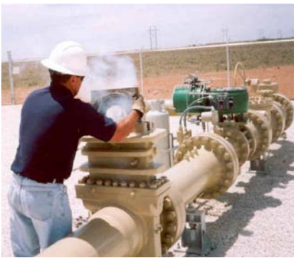
CO 2 pipeline metering
