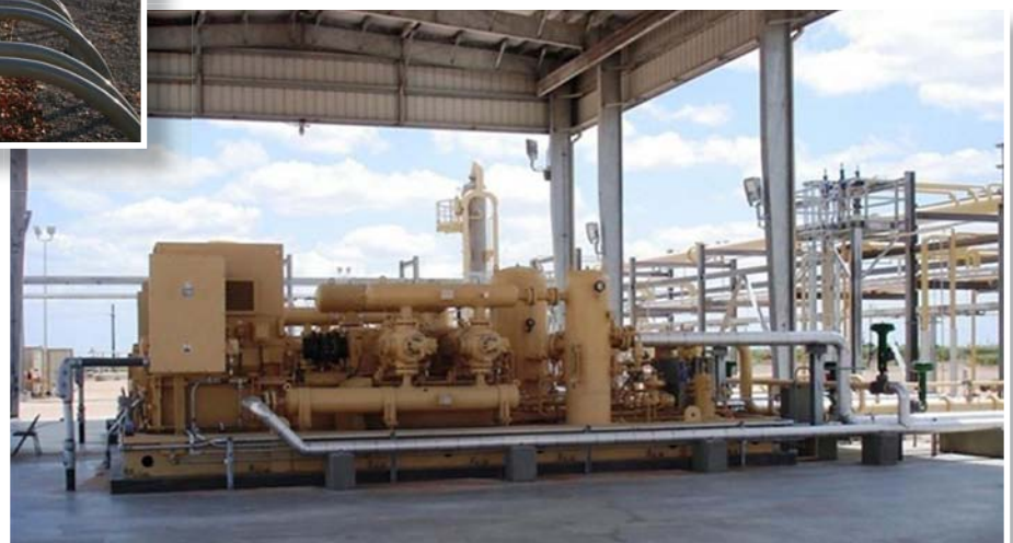
Compressor for compressing gas prior to re-injection
