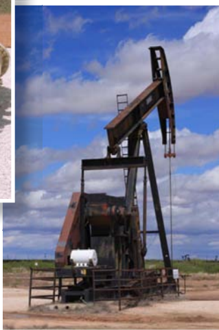
Production well pump jack
