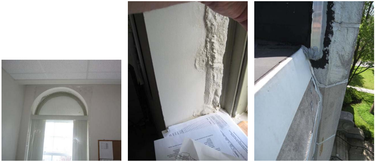
Figure 11. Moisture issues at windows in retrofitted building (Brennan 2011)
