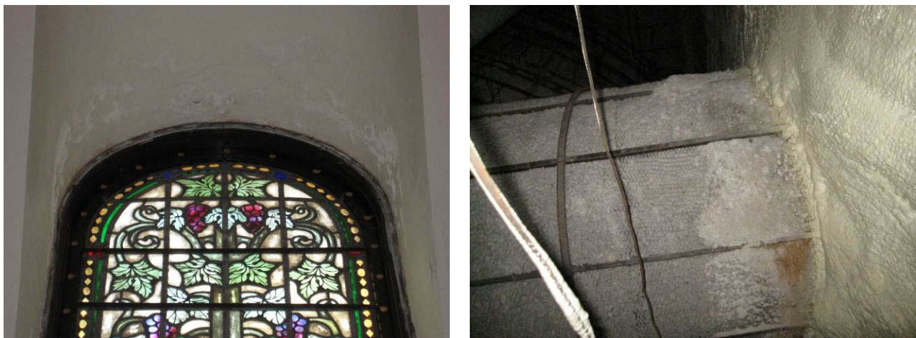
Figure 12. Moisture issues at chapel windows (Brennan 2011)
