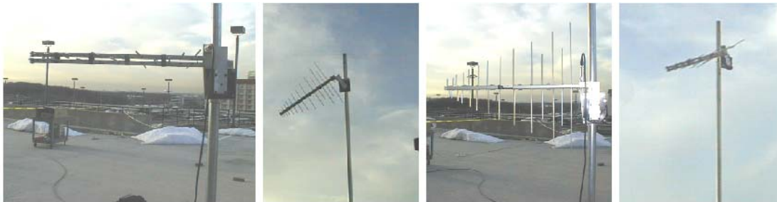
(a) Level, horizontal elements (b) Elevated, "vertical" elements (c) Vertical elements (d) Elevated, "horizontal" elements
