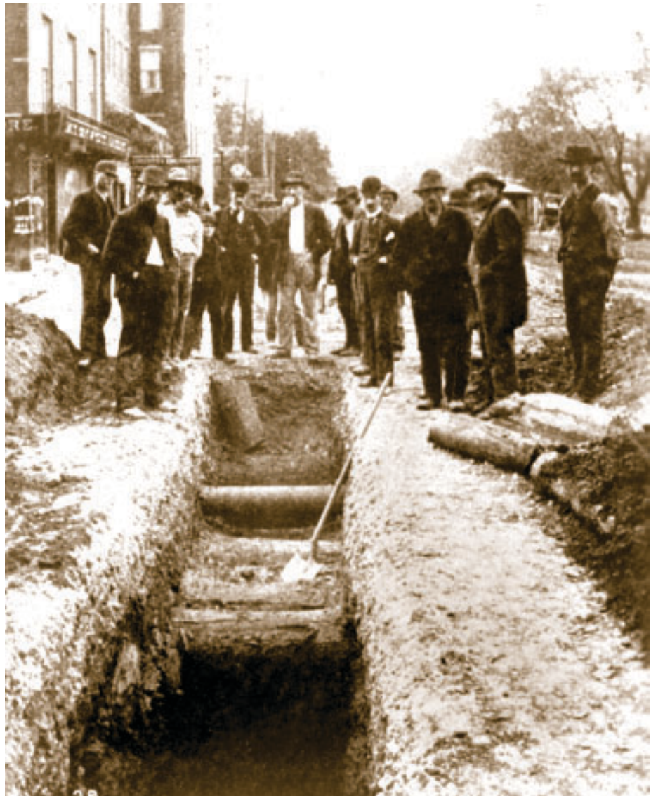
Huge logs were laid over early Dayton streets to prevent wagons and carriages from sinking in the mud. Here, some of the old “corduroy” paving is uncovered, 1890s. (Dayton Metro Library)
