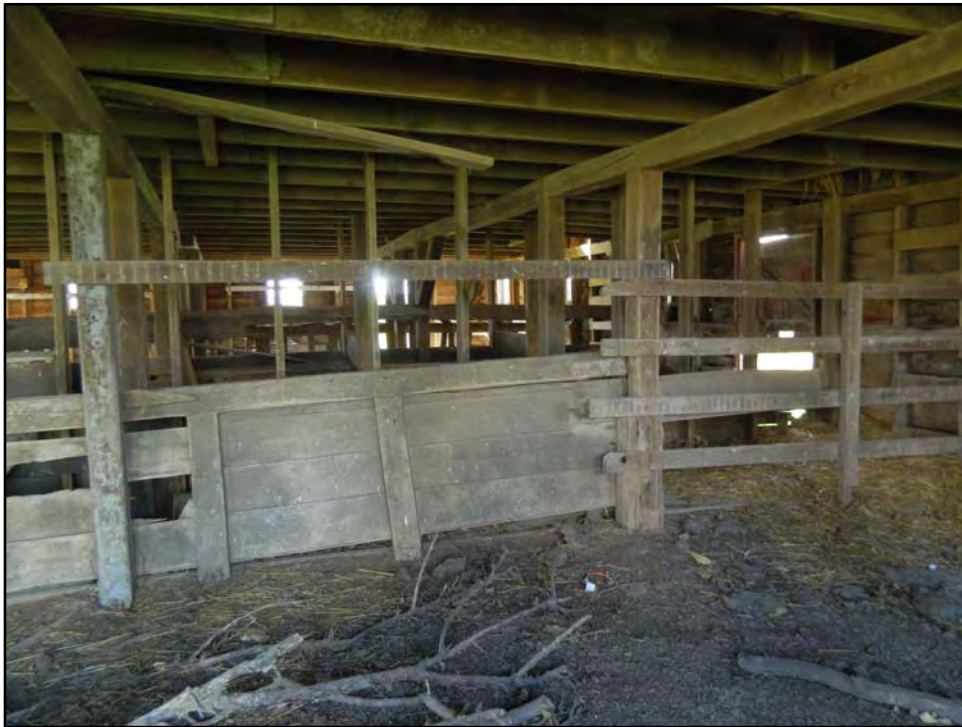
Figure 5.4. Interior of first floor of gambrel roof barn, looking west (RCG&A March 2012).
