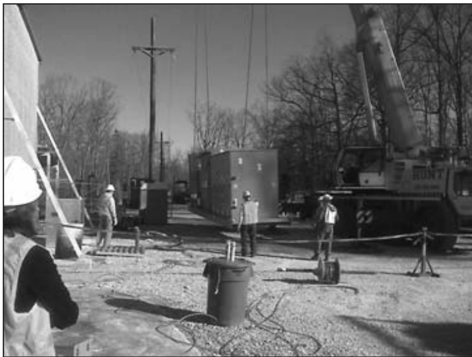
Employees from the main contractor, CH2MHill, and sub-contractor Terra-Therm provide assistance to the Dennis Hunt & Company crane guiding an electrical substation into place behind the Model Shop. This substation will soon power the thermal treatment remediation system being used to remove the PCE from this site. (Photos provided)
