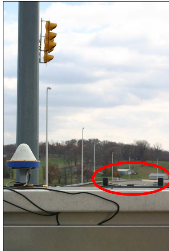
Figure 12 Wireless communications antennas (surrounded by circle).
