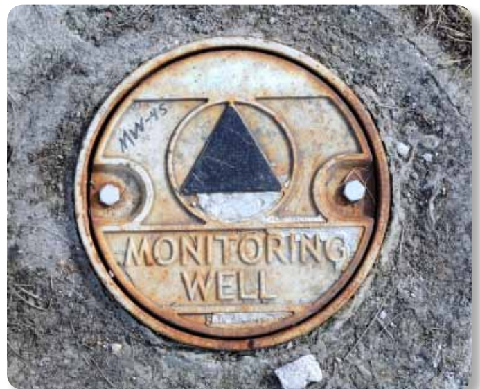
Annual groundwater monitoring is an example of a physical LUC used at Shaw A.F.B. to ensure protection of human health and the environment.
