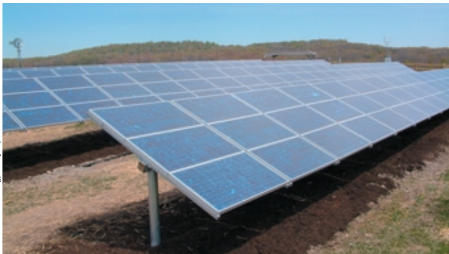
Green Mountain Energy Company installed a new solar array at Lake Farmpark, 25 miles east of Cleveland to meet the needs of the Northeast Ohio Public Energy Council (NOPEC), a buying group of nearly 100 communities in northeast Ohio.
