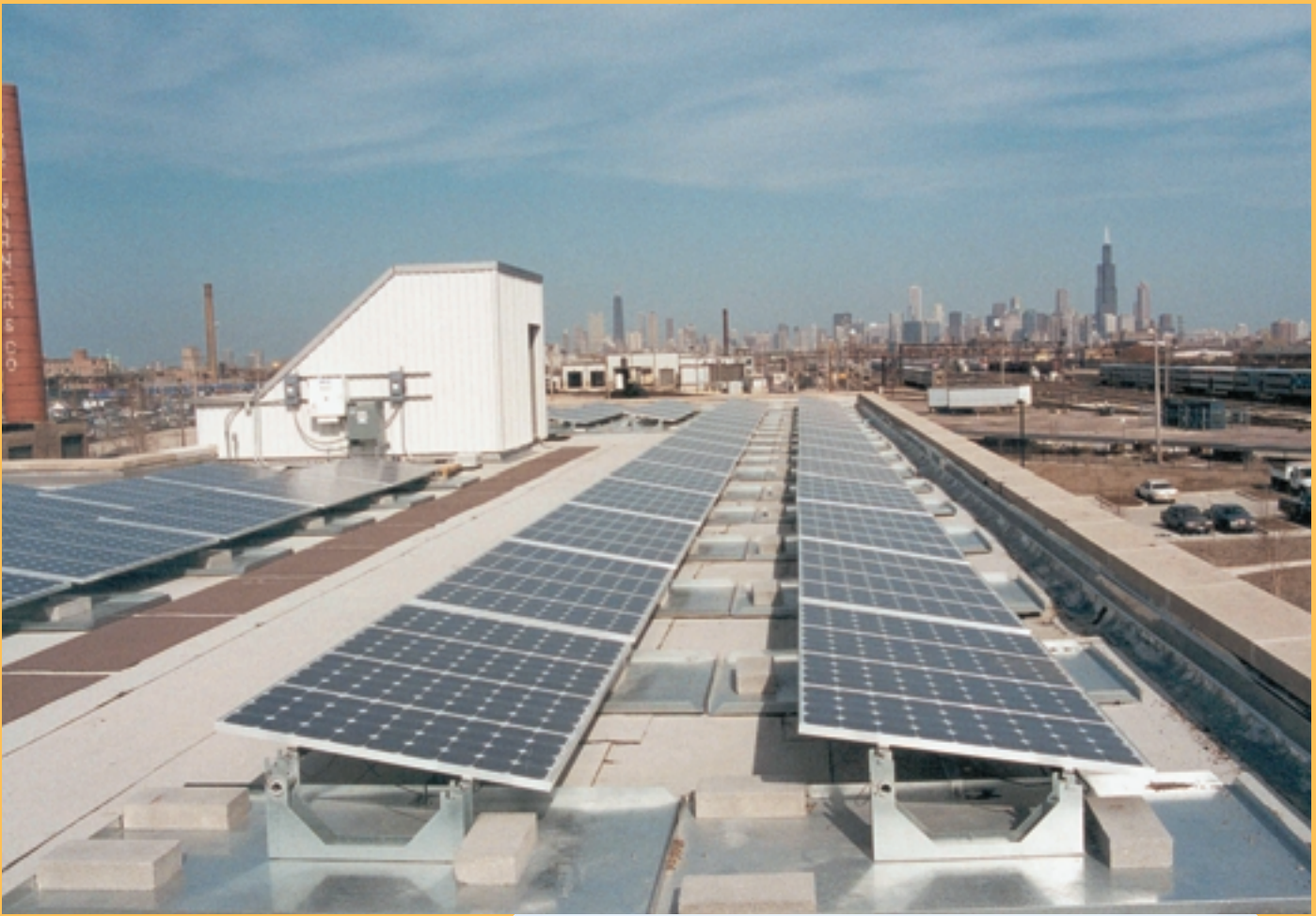
The city of Chicago has formed an alliance with 47 other local government agencies to increase their reliance on clean energy sources. As part of this effort, Chicago has installed solar electric systems on a number of the city's buildings, including the Chicago Center for Green Technology shown here.
