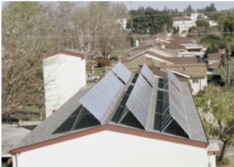
The Episcopal Church has been particularly active in spearheading the use of renewable energy technologies. For example, Christ Episcopal Church in Ontario, California, installed solar panels on their church earlier this year.
