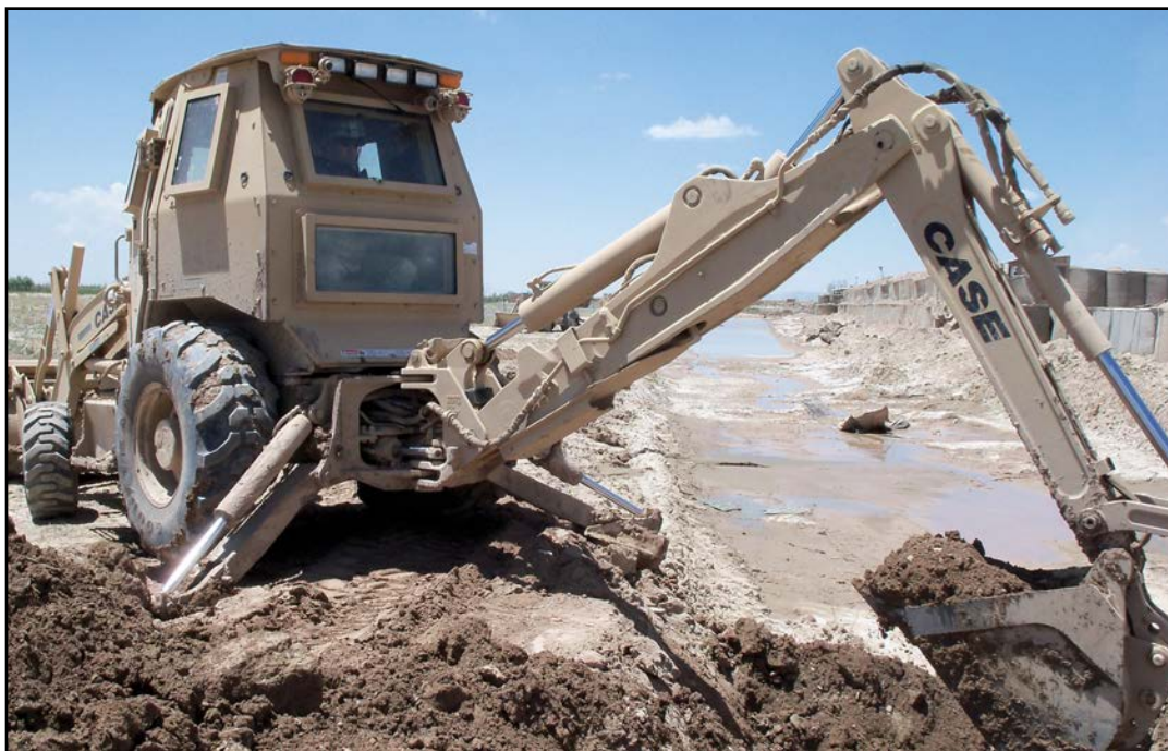
Senior Master Sgt. Nathan Colborn, 434th Civil Engineer Squadron, operates a backhoe during his recent deployment to Afghanistan. (U.S. Air Force photo)
