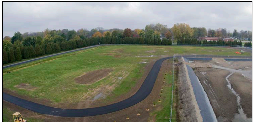
Grissom's new track, which is still under construction, is scheduled to be open for business in April 2012. (U.S. Air Force photo/Senior Airman Jami Lancette)
