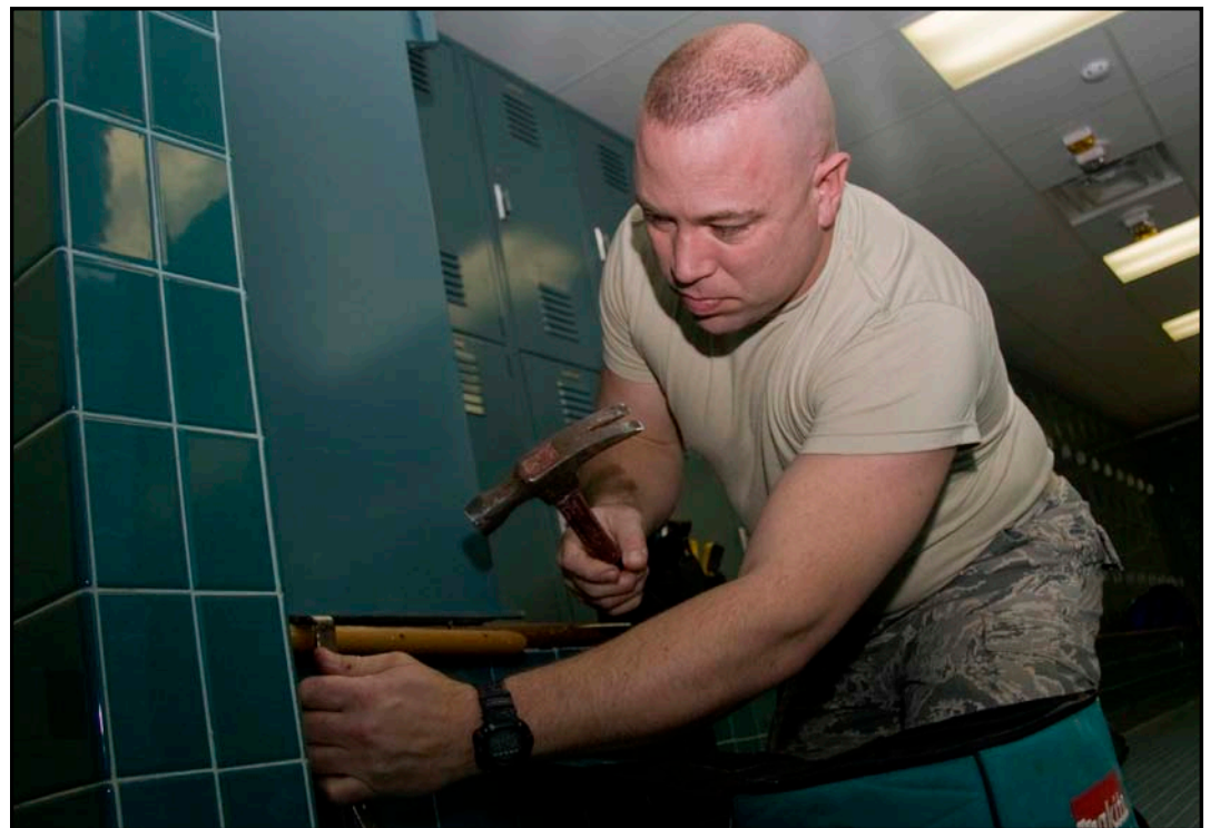
Using a hammer and crowbar, Airmen 1st Class David Kessen, 434th Civil Engineer Squadron engineer apprentice, persuades a group of old lockers loose as he removes them from the base fitness center recently. New wooden lockers were recently installed, which provide double the storage space to the user and replaced aging metal lockers that were originally installed when the facility was a child development center.
