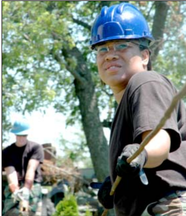
Staff Sgt. Soyica Hinkle, an electrical systems craftsman with the 434th Civil Engineering Squadron, pulls a cable used to hoist a telephone pole into position behind Bldg. 671. During the July unit training assembly, the civil engineers set poles to use for future training programs.
