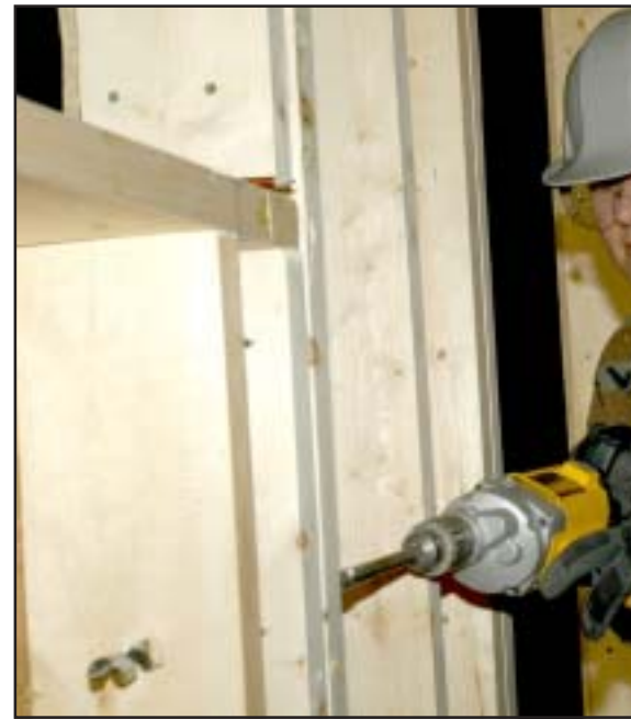
Senior Airman Rebecca Aldrich, a power production apprentice, drills a hole to run electrical lines during the home construction.
