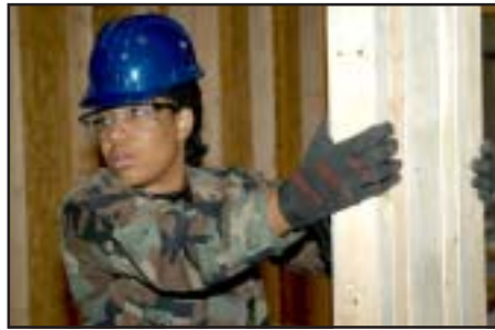
Senior Airman Soyica Hinkle, an electrical systems apprentice, holds a newly erected wall in place until it is secured.
