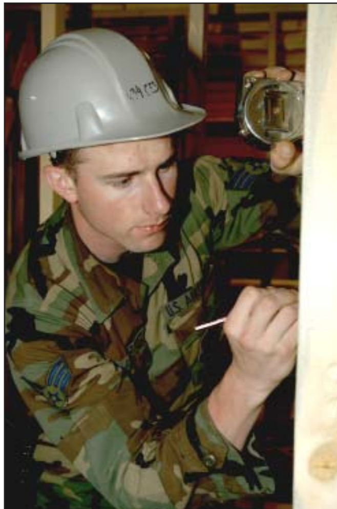
Senior Airman Michal Bednarczyk, an electrical systems apprentice, marks the location where a light switch will be installed.
