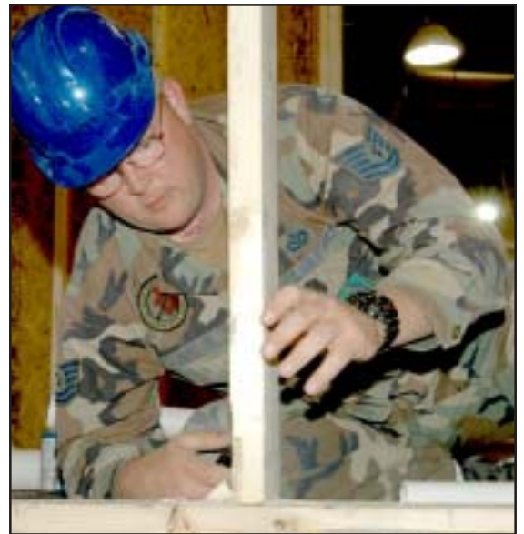
Above, Tech. Sgt. Chris Heston, a utilities systems journeyman, maps out the plumbing in the bathroom of the construction project.
