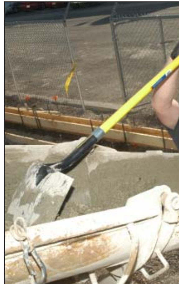
Tech. Sgt. Steven Wolf, a heavy equipment operator, works on the chute as he and other CES members build a house at an Indian Foundation worksite.
