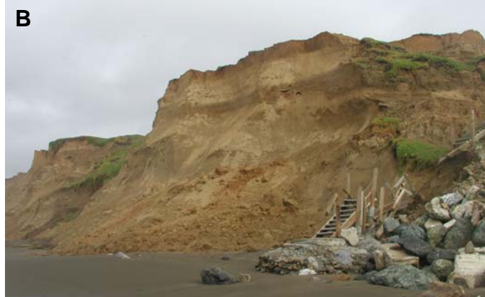
Figure 4. Schematic diagram (A) and photo (B) of weakly cemented coastal cliff failure mode. The failure surface is typically inclined at 65° to the horizontal.
