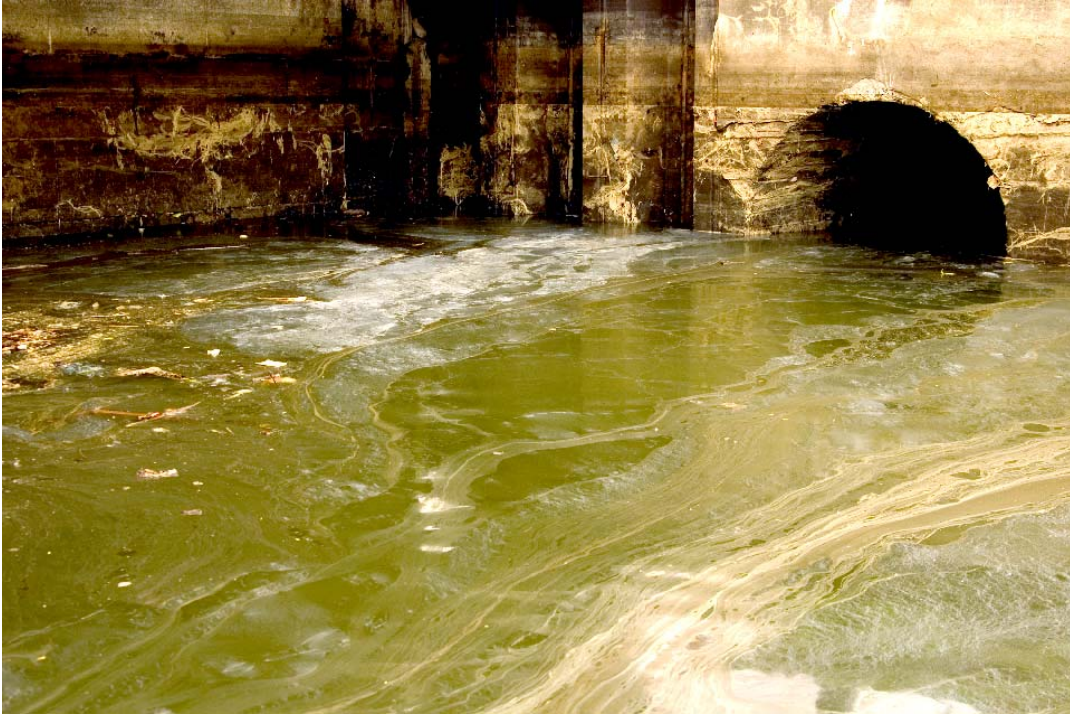
Overflow pipes like this one on Newtown Creek discharge raw sewage and dirty stormwater into New York Harbor. Image: Giles Ashford © 2004.
