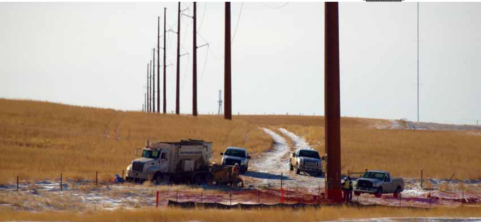
Construction on the Montana Alberta Tie Limited Project continues about 5 miles north of Cut Bank, Mont.
