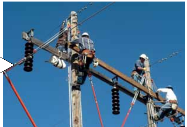
Western linemen use needed crossarm change-out work on the Canyon Ferry-East Helena 115-kV lines as an opportunity for hot stick training.
