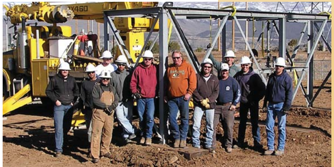
Line crews from Montrose, Cheyenne and Phoenix combined efforts to install a shoo-fly for Tri-State Generation and Transmission.
