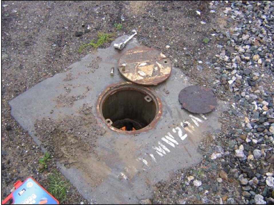
Well IR07MW20A1; Well is in good condition , 1 bolt needs repair, well is locked with no water in vault . Photo orientation - North Date 10 Jan 08
