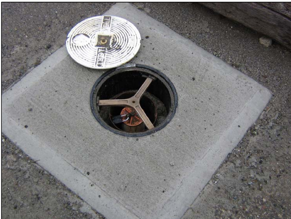
IR26MW40A; Well in good condition, locked with water in the vault. Photo orientation - South Date 09 Jan 08
