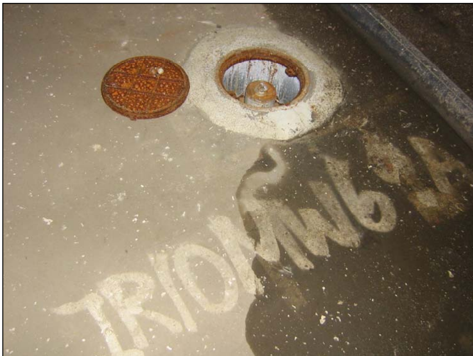
Well IR10MW69A; Well is in good condition, is not locked and there is no water in vault. Photo orientation - North Date 09 Jan 08
