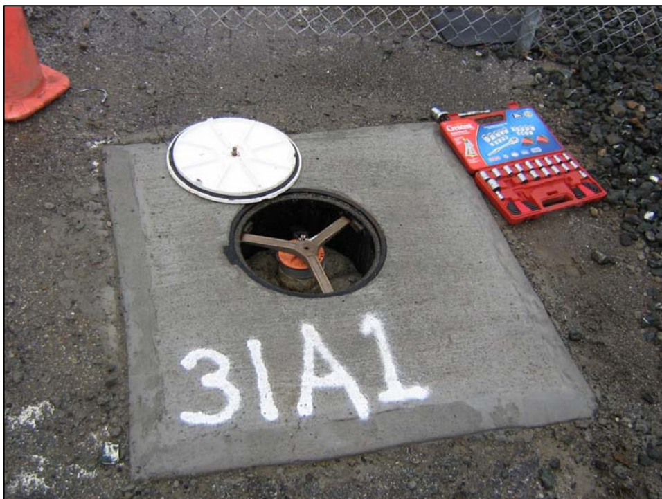
IR10MW31A1; Well is in good condition and locked and there is no water in the vault. Photo orientation - South Date 10 Jan 08
