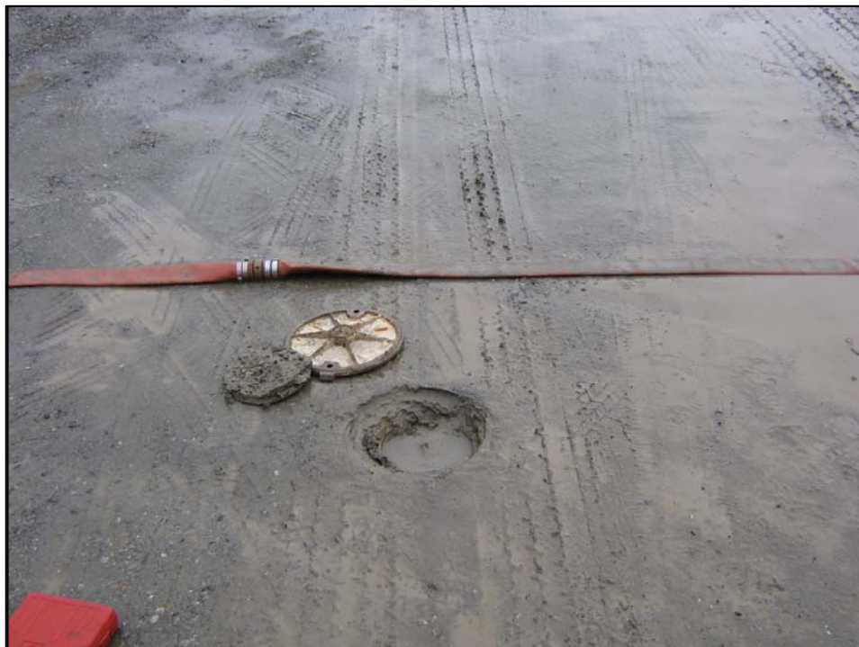
Well IR62MW07A; Well is in poor condition with no bolts, locked, and no water in vault. Photo orientation - North Date 10 Jan 08
