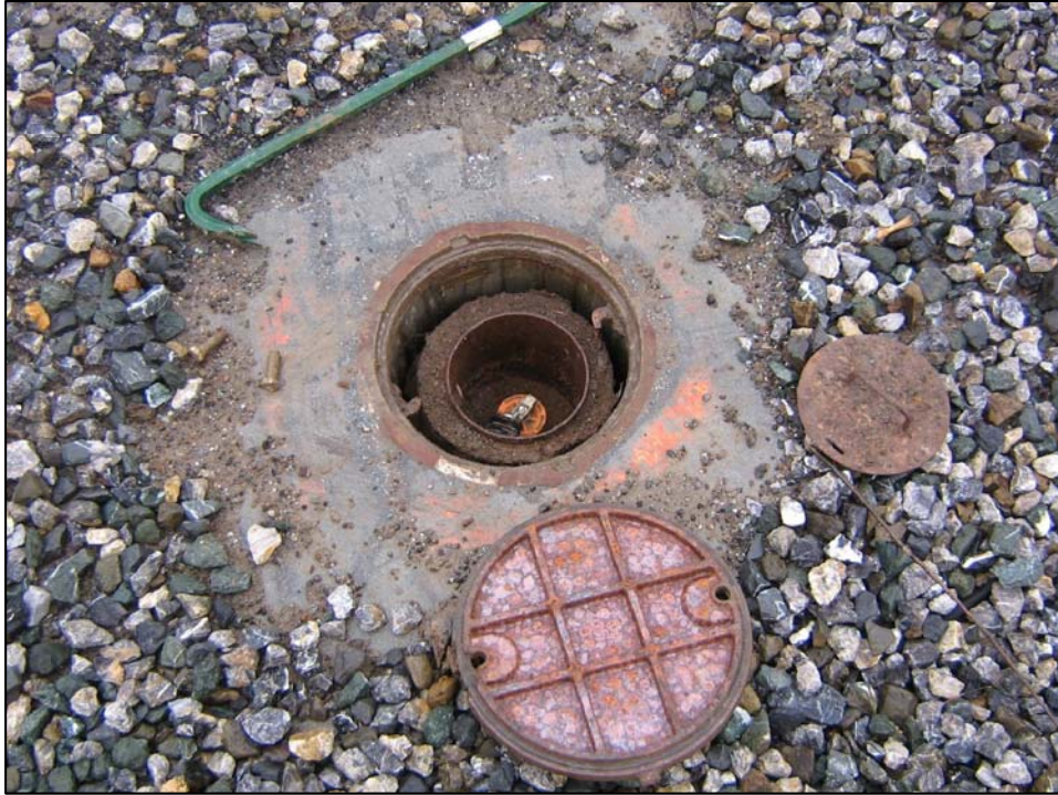
Well IR07MW20A; Well is in good condition with bolts stripped, locked and there is no water in vault. Photo orientation - North Date 10 Jan 08
