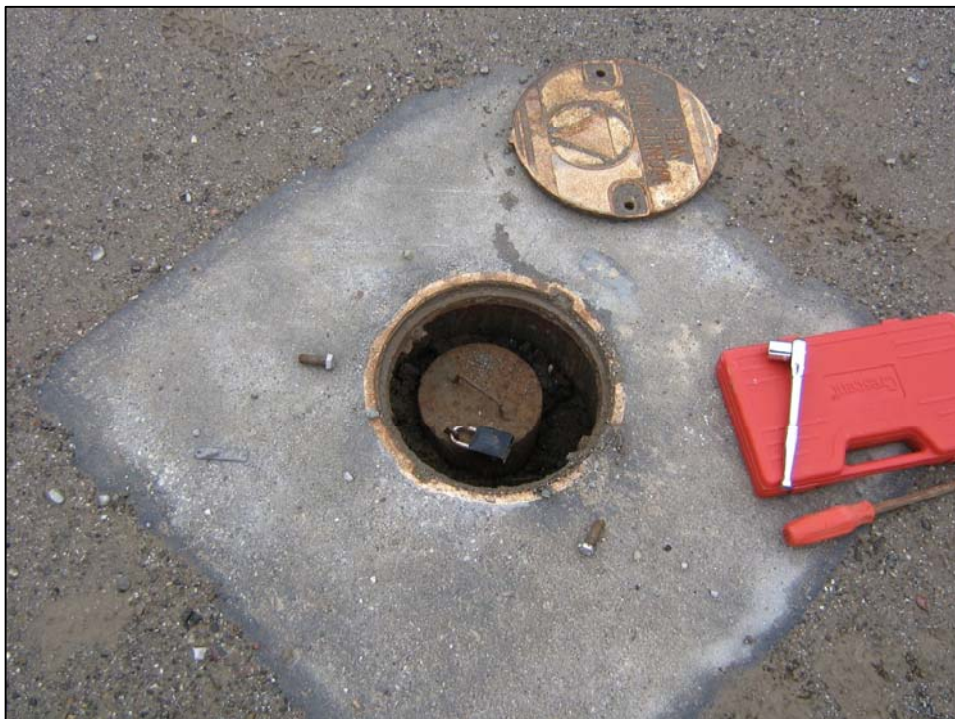
Well IR10P13A; Well is in good condition, locked and there is no water in vault. Photo orientation - North Date 09 Jan 08
