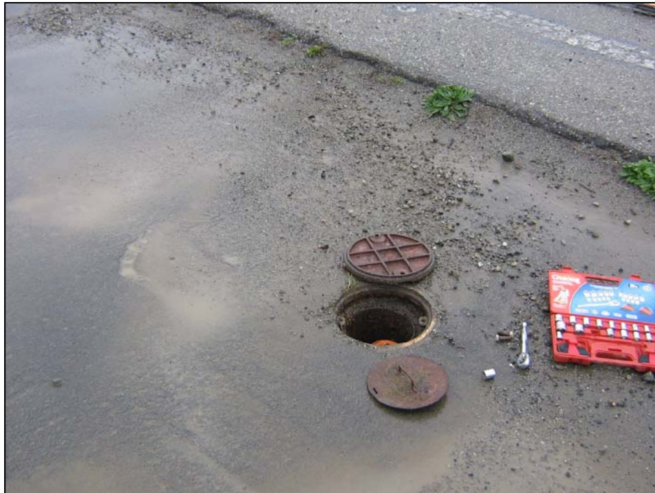
Well IR46MW48A; Well is in good condition, locked and there is no water in vault. Photo orientation - North Date 10 Jan 08
