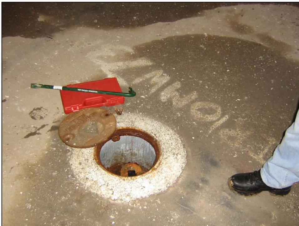
Well IR10MW73A; Well is in good condition, locked, and there is water in vault. Photo orientation - South Date 09 Jan 08
