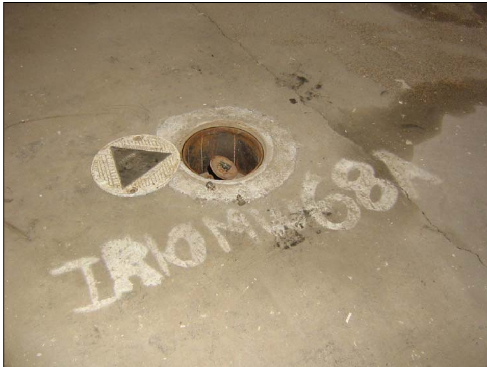
Well IR10MW68A; Well is in good condition but the cap does not fit right, not locked and no water in vault. Photo orientation - South Date 09 Jan 08
