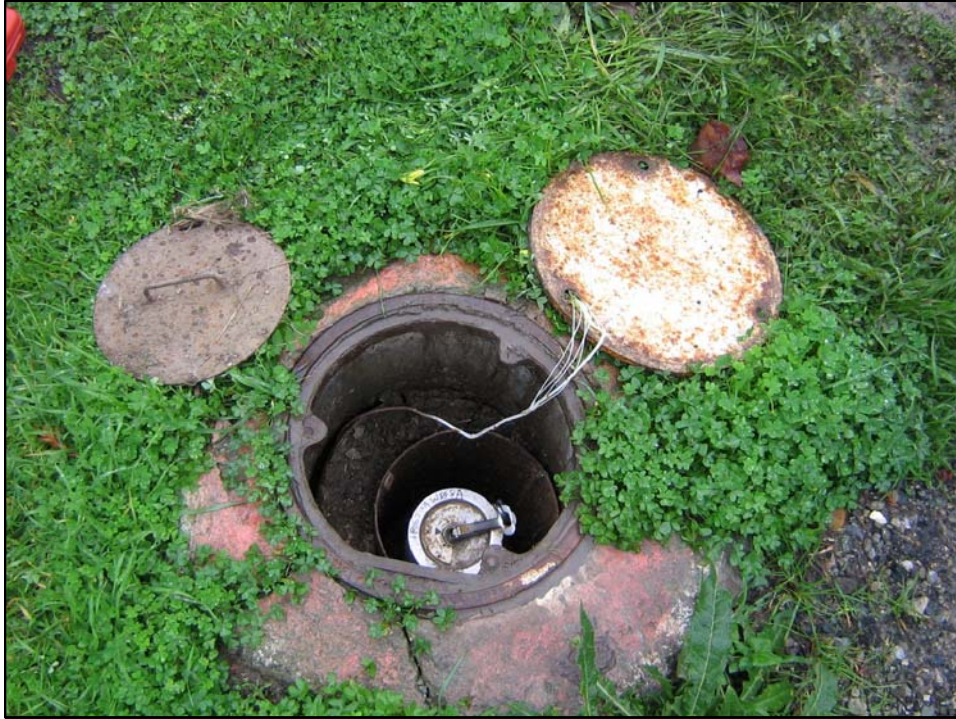
Well IR62MW08A; Well is in good condition with no bolts, locked, and there is no water in vault. Photo orientation - North Date 10 Jan 08
