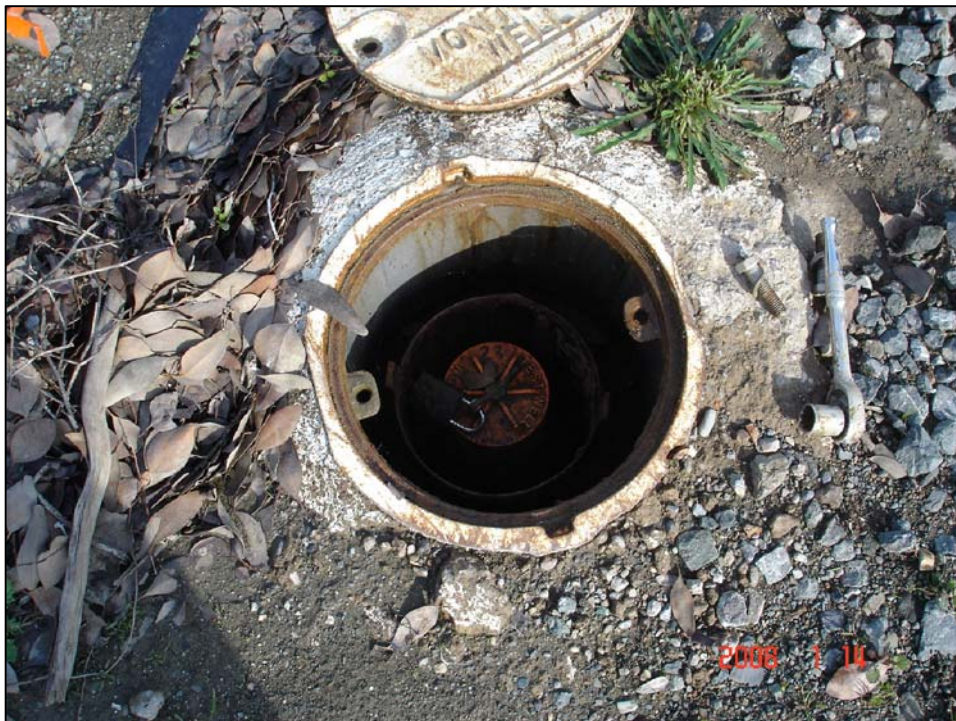
Well IR07MW23A; Well is in good condition, locked, and there is no water in vault. Photo Orientation - East Date 14 Jan 08
