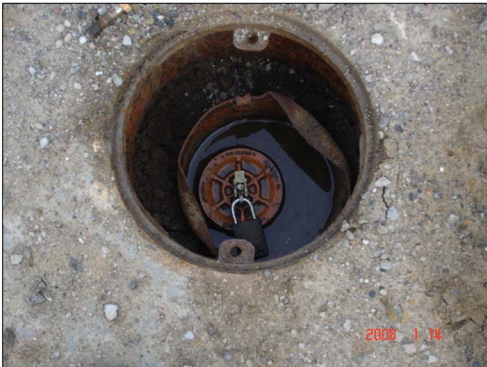
Well IR25MW44A; Well is in poor condition, casing is bent, locked, and there is water in vault
