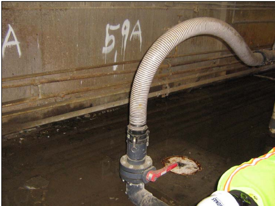
Well IR10MW59A; covered in water. Photo orientation - South Date 09 Jan 08
