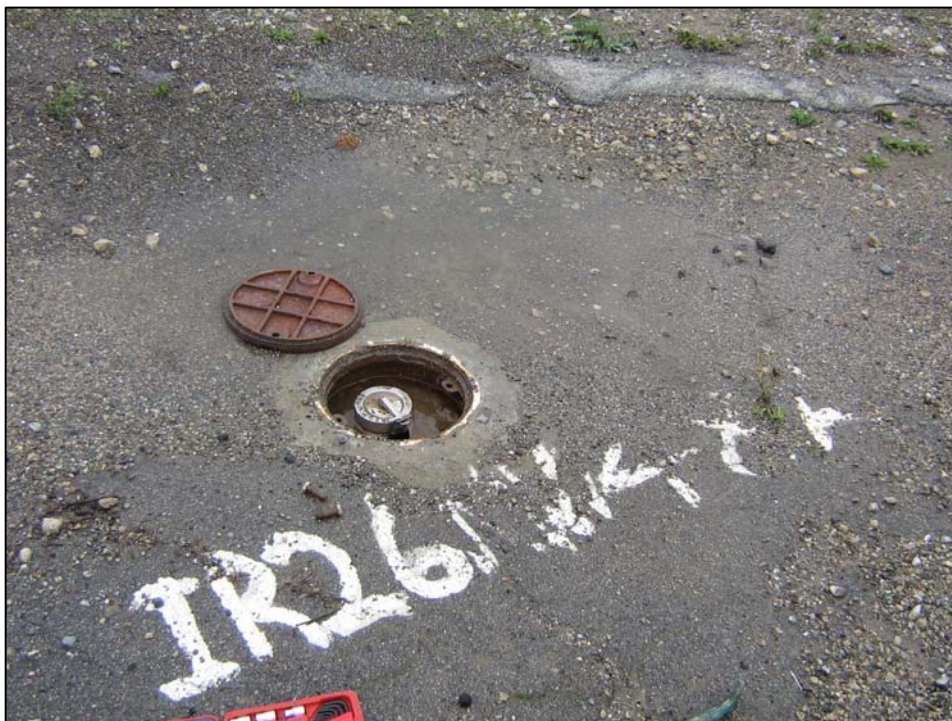
Well IR26MW48A; Well is in good condition, locked and water in vault. Photo orientation - North Date 10 Jan 08
