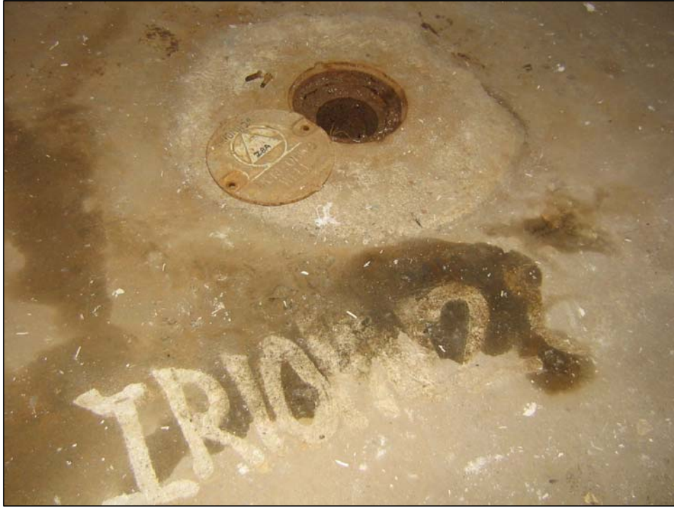
Well IR10MW28A; Well is in good condition, locked, and no water in vault. Photo orientation - West Date 09 Jan 08
