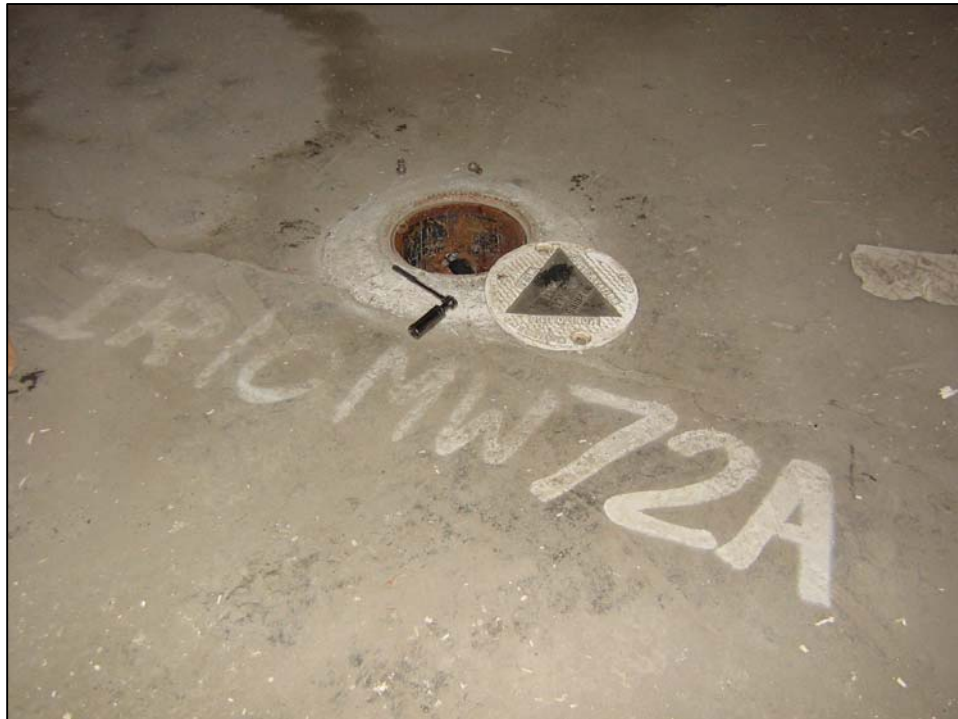
Well IR10MW72A; Well is in good condition, locked, and no water in vault. Photo orientation - North Date 10 Jan 08
