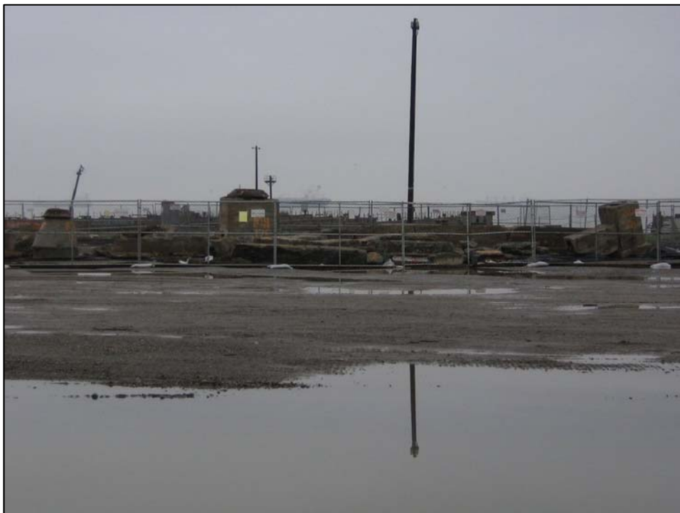
Photo is of excavated sewer lines and storm drains. All excavations in Parcel B are properly fenced with warning signs posted. Photo Orientation - North Date 9 Jan 08
