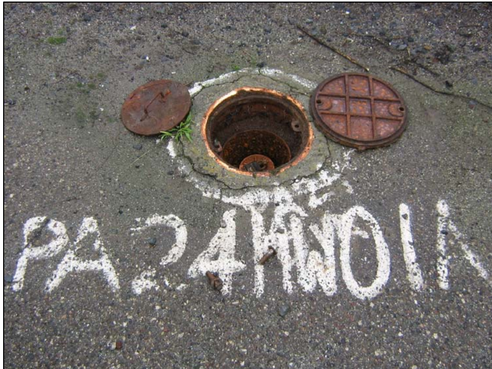
Well PA24MW01A; Well is in good condition, locked and there is water in vault. Photo orientation - East Date 10 Jan 08
