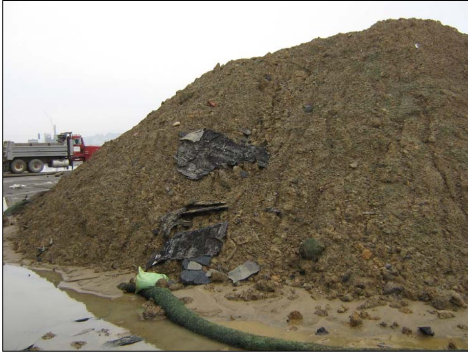
Photo is of stock piled earth treated with "Super Snot". "Super Snot" is an adhesive that prevents contaminated soils from washing away during rains.
