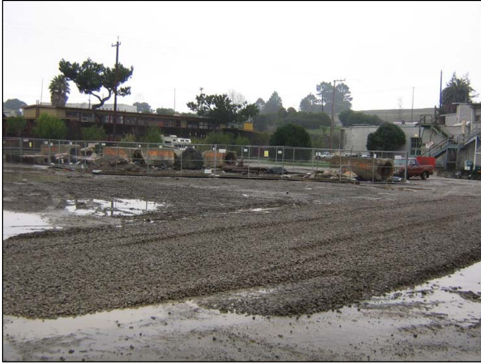
Photo is of drainage rock laid down to prevent pooling of surface water on streets. Drainage rock has been laid down in low areas along roads to increase access. Photo Orientation - South Date 9 Jan 08
