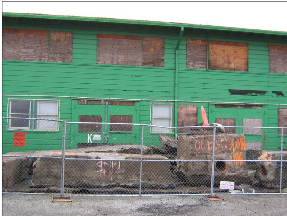
Photo is of secured building. All unoccupied buildings in Parcel B are secured. Photo Orientation - West Date 9 Jan 08
