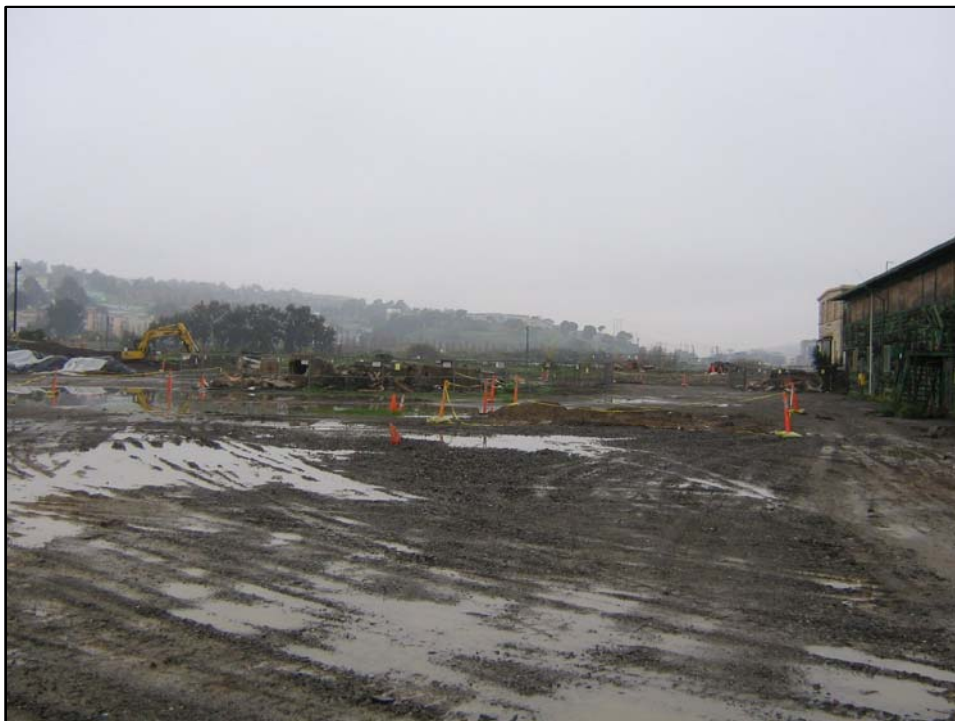
Photo is of general site condition and shows, former excavation, current excavation, excavated material, road conditions and drainage rock. Photo Orientation - West Date 9 Jan 08
