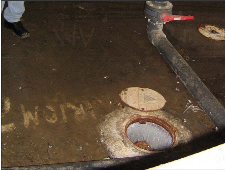
Well IR10MW74A; Well is in good condition, locked, with no water in vault. Photo orientation - South Date 09 Jan 08
