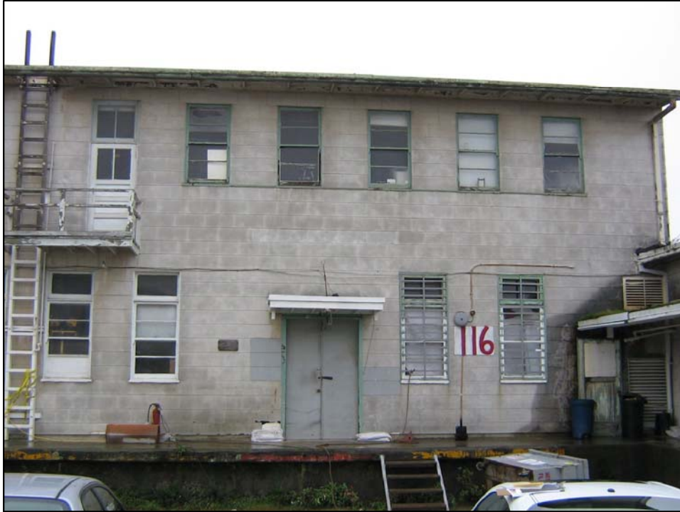
Photo of building 116 which contains artist studios, all buildings with artist studios are in good condition. Photo Orientation - West Date 9 Jan 08
