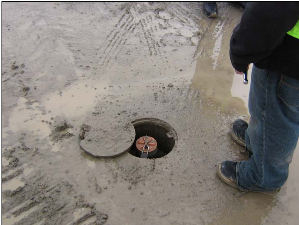
Well IR10MW63A; Well is in poor condition with cover broken, well is locked and there is water in vault. Photo orientation - South Date 09 Jan 08
