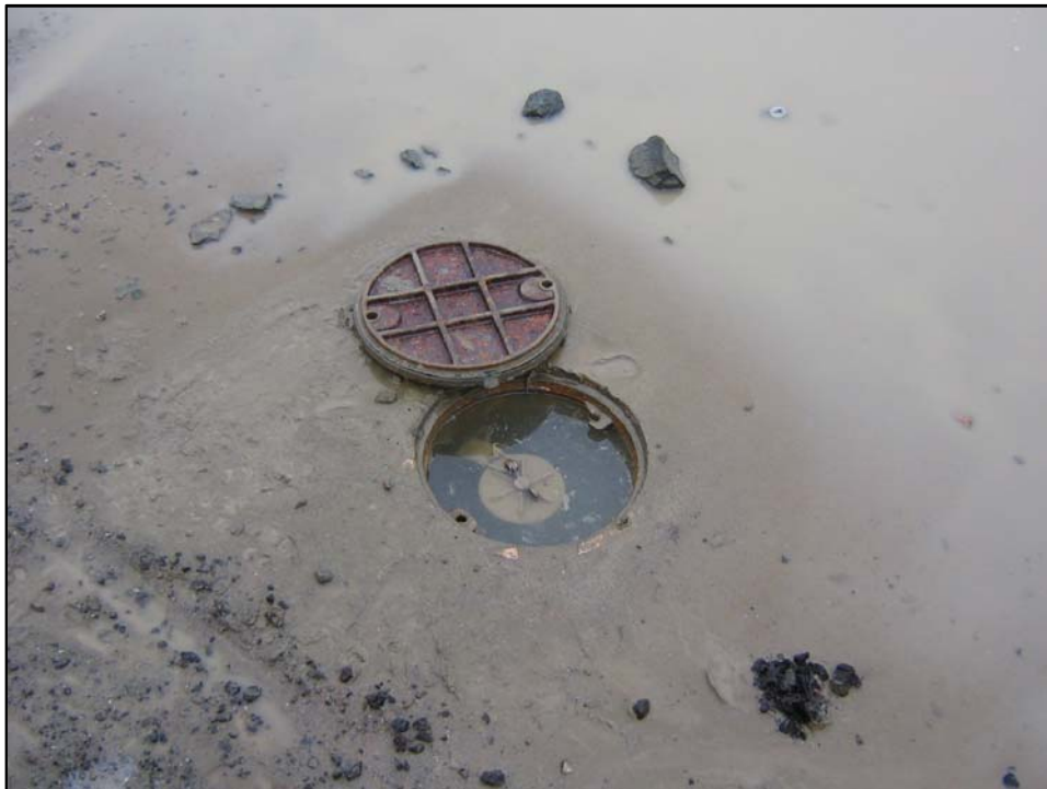
Well IR25MW61A1; Well is in good condition, locked. and there is water in vault Photo Orientation - North Date 10 Jan 08
