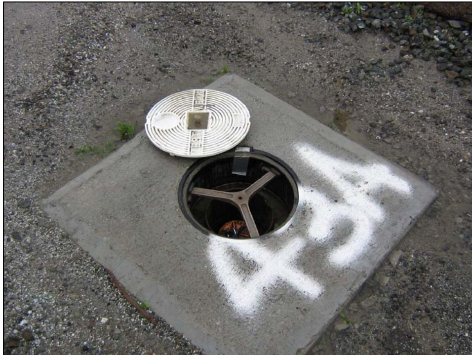
Well IR26MW43A; Well is in good condition, locked, with water in vault. Photo orientation - North Date 10 Jan 08
