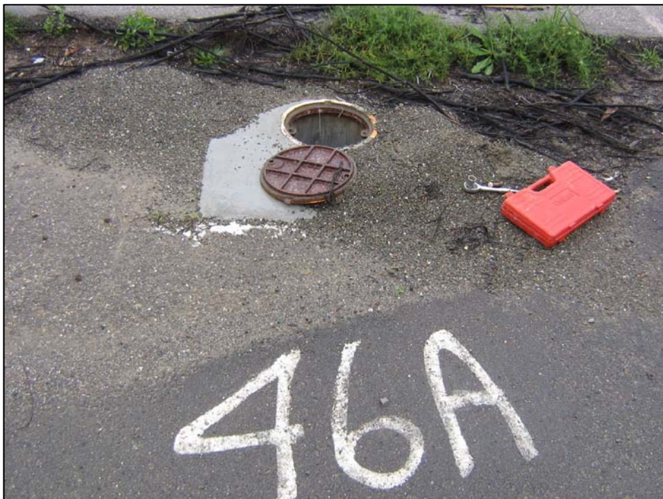
Well IR46MW46A; Well is in good condition, locked, and no water in vault. Photo orientation - East Date 10 Jan 08
