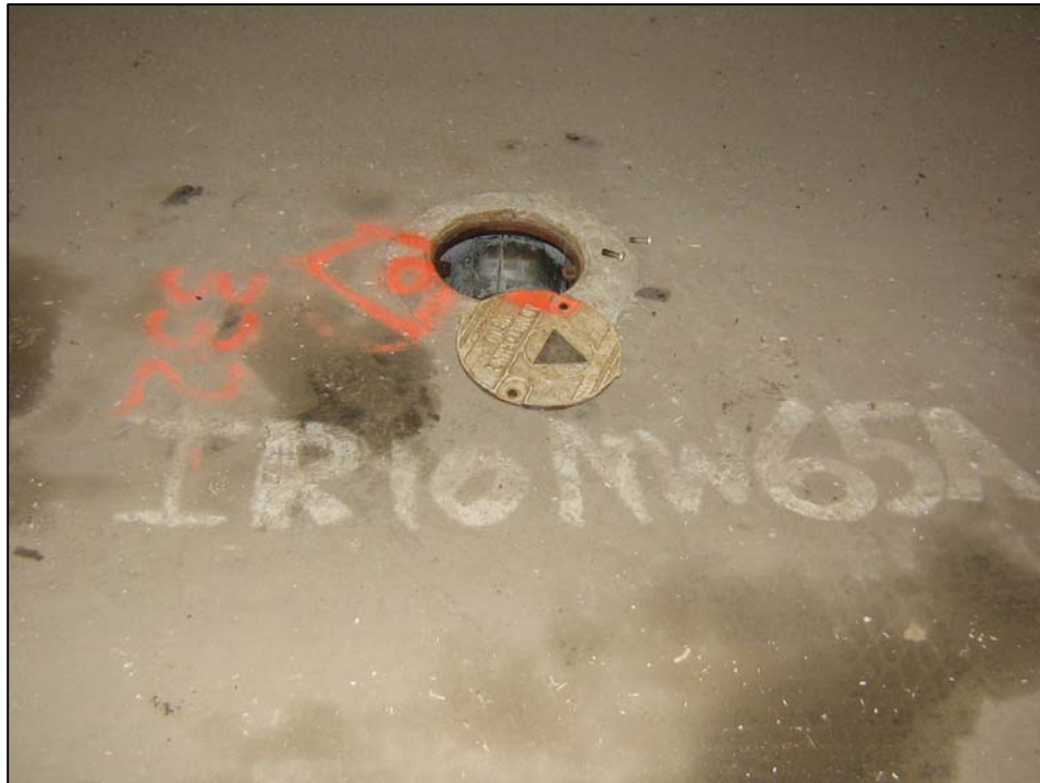
Well IR10MW65A; Well is in good condition, locked, and no water in vault. Photo orientation - West Date 10 Jan 08
