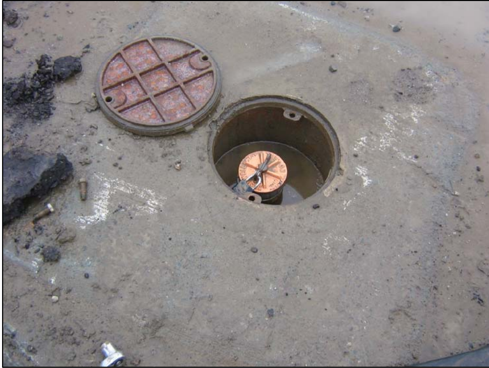
Well IR25MW61A2; Well is in good condition, locked and there is water in vault. Photo orientation - South Date 09 Jan 08
