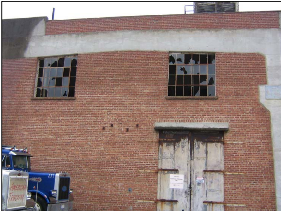
Photo is of broken windows. Photo is representative of broken windows in Parcel B. Photo Orientation - South Date 9 Jan 08
