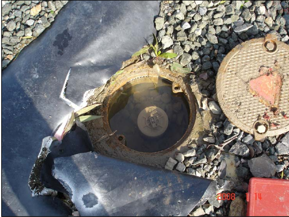
Well IR07MW27A; Well is in good condition, unlocked, and there is water in vault Photo Orientation - East Date 14 Jan 08
