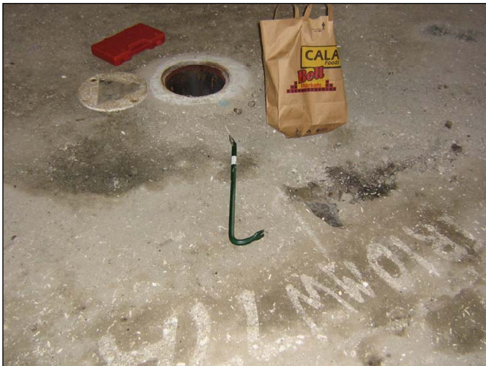
Well IR10MW77A; Well is in good condition, locked and there is no water in vault. Photo orientation - South Date 09 Jan 08
