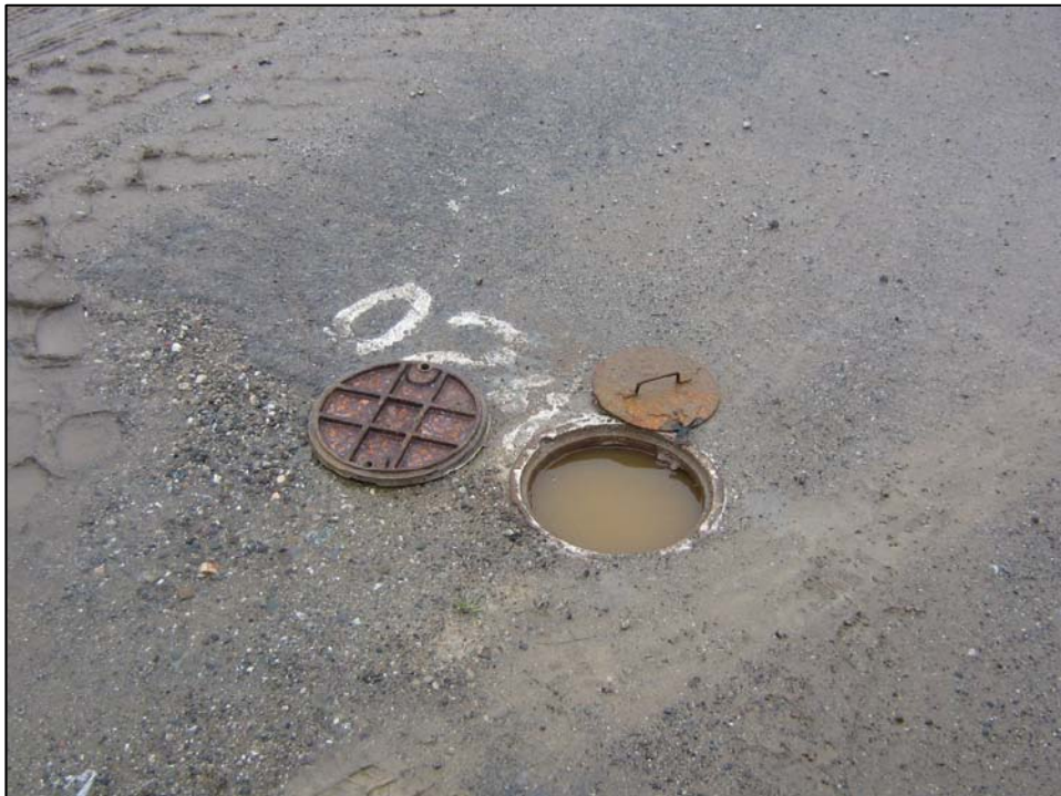
Well PA50MW02A; Well is in good condition with no bolts, it is not known if locked, and there is water in vault. Photo orientation - North Date 10 Jan 08
