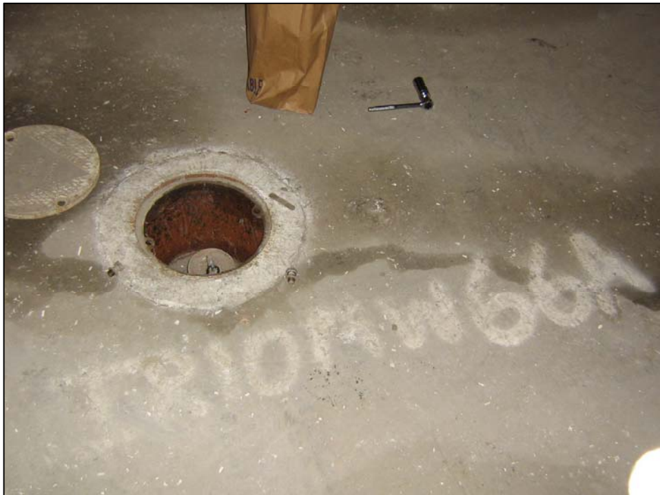
Well IR10MW66A; Well is in good condition, locked, and no water in vault. Photo orientation - North Date 09 Jan 08
