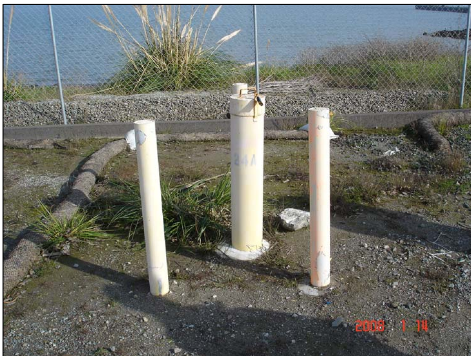
Well IR07MW24A; Well is in good condition, and locked. Photo Orientation - East Date 14 Jan 08
