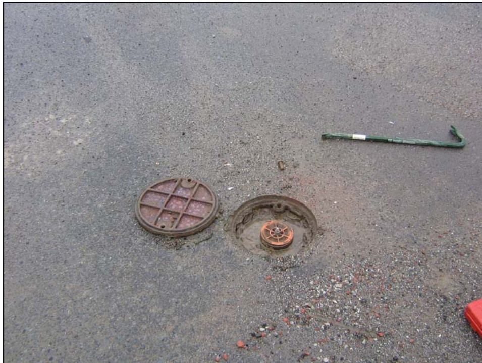
Well IR24MW05A; well in good condition, well is not locked and there is water in vault. Photo orientation - North Date 10 Jan 08
