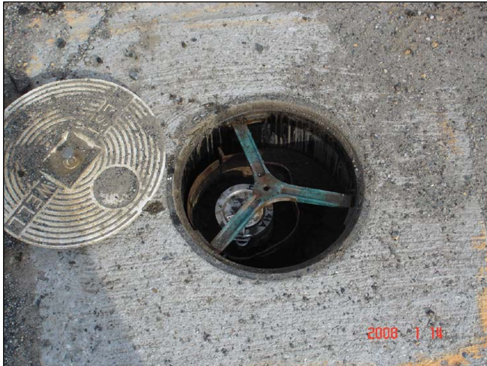
Well IR25MW41A; Well is in good condition, unlocked, and there is water in vault. Photo Orientation - East Date 14 Jan 08
