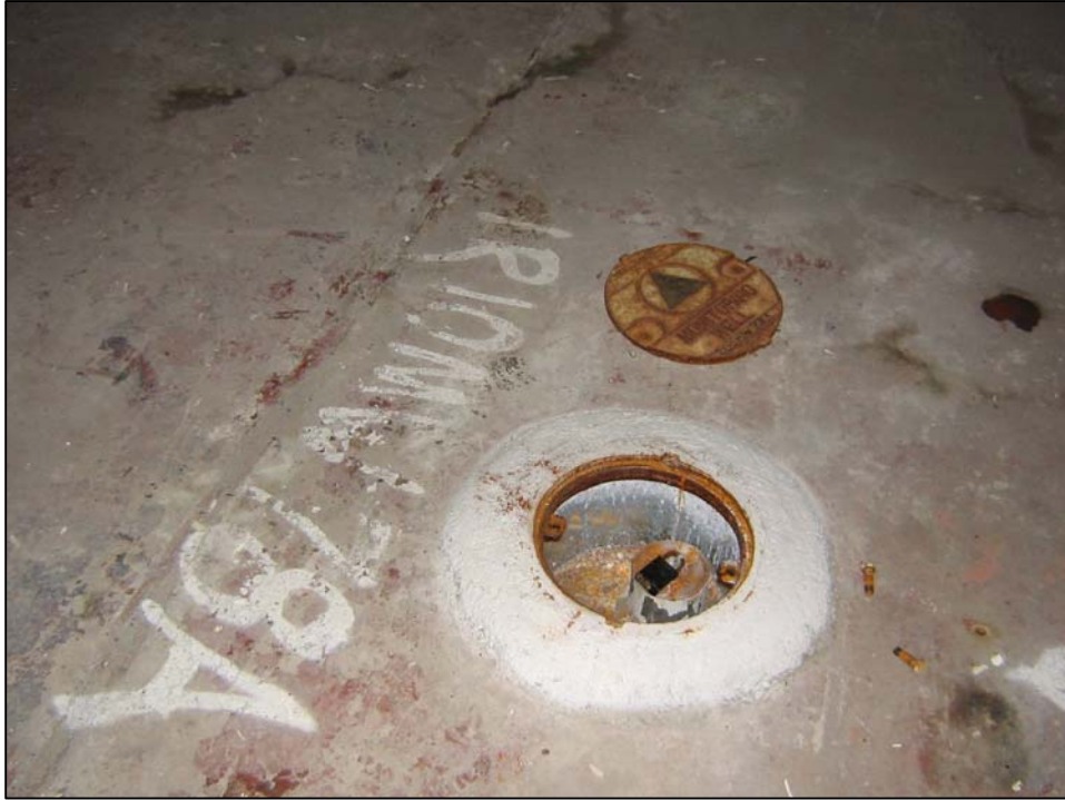
Well IR10MW78A; well is in good condition, locked with no water in vault. Photo orientation - South Date 09 Jan 08
