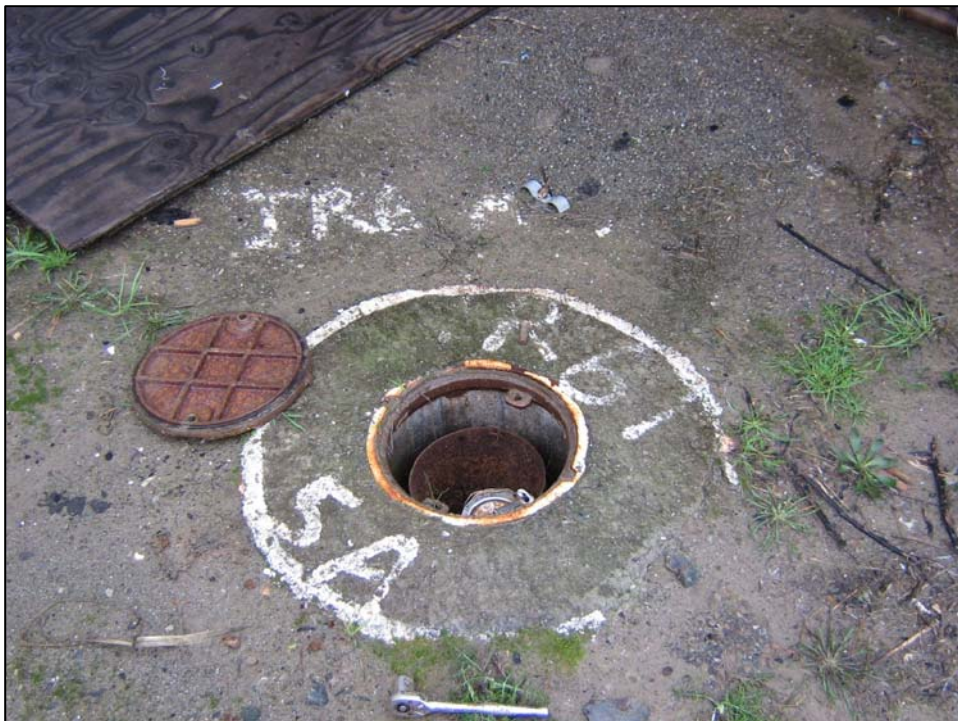
Well IR16MW04A; Well is in good condition, missing bolt, locked and water in vault. Photo orientation - North Date 10 Jan 08
