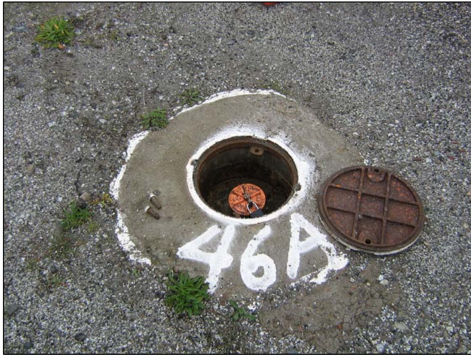
Well IR26MW46A; Well is in good condition, bolt eyelet broken, and locked. Photo orientation - North Date 10 Jan 08
