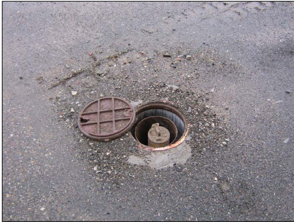
Well IR10MW05A; Well cover cracked, well is locked and there is water in vault. Photo orientation - East Date 10 Jan 08
