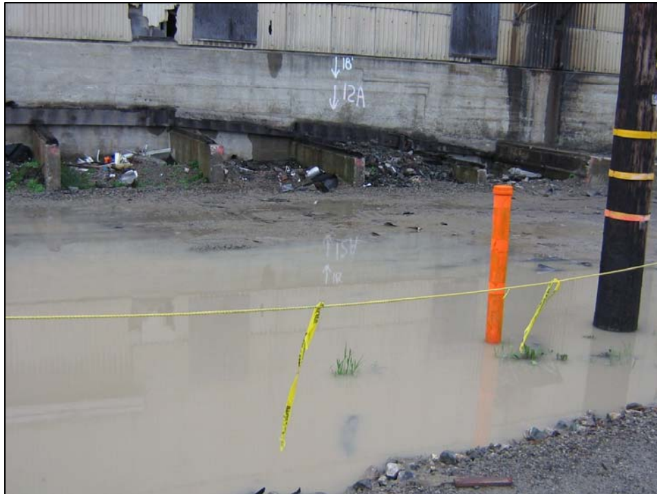
Well IR10MW82A; Well is covered with water. Photo orientation - South Date 09 Jan 08
