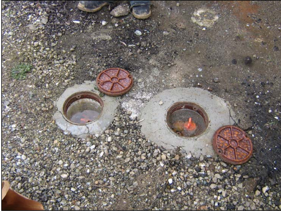
(2) Unidentified Wells; wells in good condition, not locked, water in vault, no name. Photo orientation - South Date 09 Jan 08
