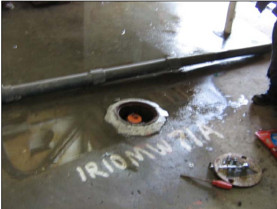
Well IR 10MW71A; Well is in good conditon, locked, and water in vault. Photo orientation - North Date 09 Jan 08
