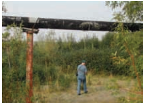
Asbestos piping is elevated, but other asbestos waste is found throughout the BIA Administrative site. D. Rudis/USFWS photo
