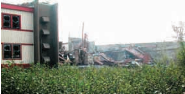
The BIA Administrative Site buildings contained asbestos, and many were partially burned in vandalism activities. D. Rudis/USFWS photo
