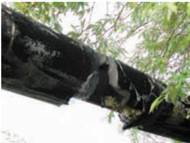
Asbestos waste, including piping, is found throughout the BIA Administrative site. D. Rudis/USFWS photo
