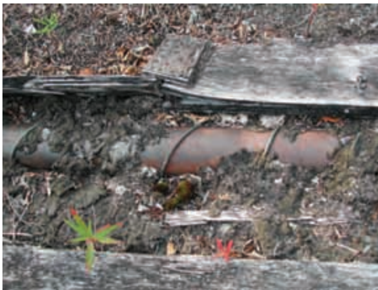
BIA Administrative site building debris and buried pipe are typical hazardous materials found on site. D. Rudis/USFWS photo
