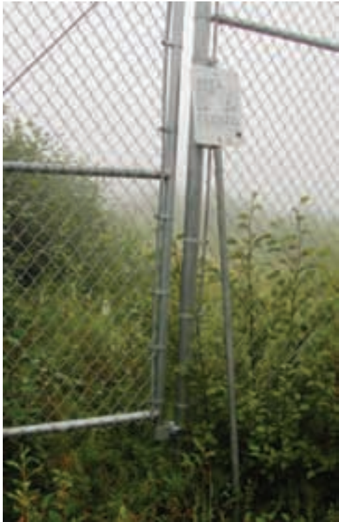
Exclusion fencing and signage around the closed BIA site sewage lagoon is inadequate to prevent trespass. D. Rudis/USFWS photo
