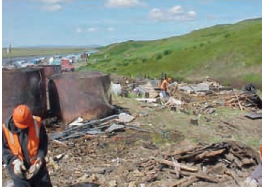
Nightmute School cleanup project in 2002 included removal of asbestos-containing materials, building and tank farm demolition, and other waste removal. Engineering/USFWS photo
