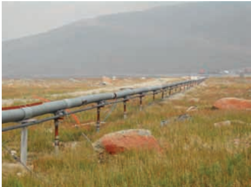
Pipelines at the Cape Romanzof LRRS carried fuel to the facility. D. Rudis/USFWS photo
