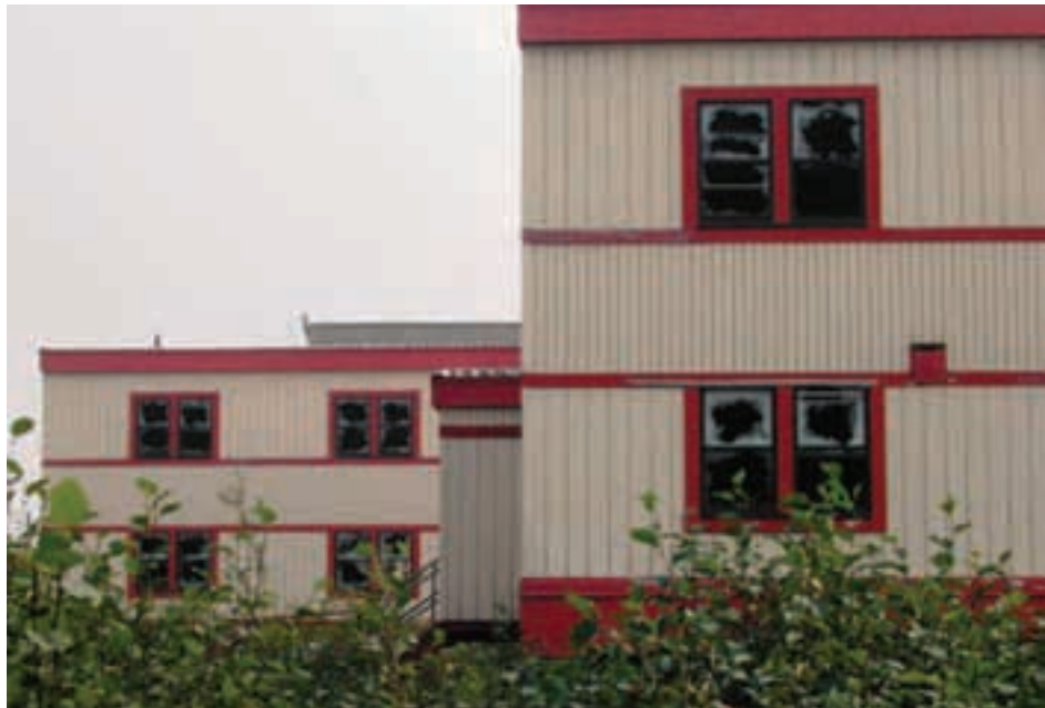
Buildings and other structures at this site pose safety and hazardous waste dangers. D. Rudis/USFWS photo
