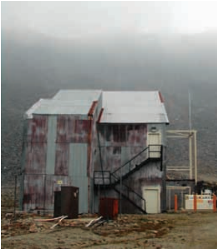
The former tramway building at the Cape Romanzof LRRS has PCB-contaminated paint and friable asbestos. PCBs and petroleum based lubricating oil were used on tramway cables. D. Rudis/USFWS photo
