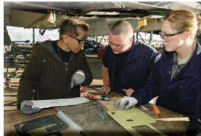
Mr. Binh Tran (l), 309 AMARG 577 CMRS; SrA Sean Carroll, 74th AMU, Moody AFB, Ga.; and SrA Christina O'Gara, 57 AMXS, Nellis, AFB, Nev., perform repairs on an A-10 wing.
