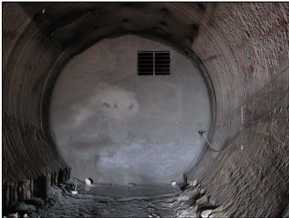
Figure 6-18. Completed bat gate in the extension drift of N Tunnel with plastic sheeting on ground below (Photo taken by D. B. Hall, February 8, 2007)
