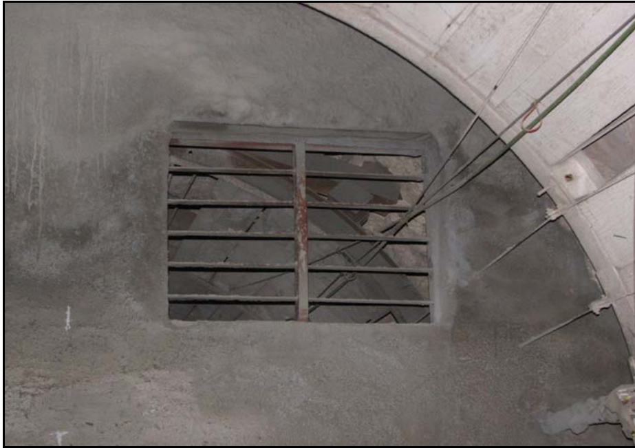
Figure 6-17. Completed bat gate in the main drift of N Tunnel (Photo taken by D. B. Hall, February 8, 2007)
