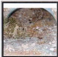
Burrow A Culvert (Inaccessible Area) Aspect: 270° (W) Height: 13 cm Width: 33 cm
