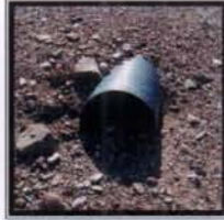
Burrow G Culvert Aspect: 340° (NE) Height: 15 cm Width: 43 cm
