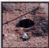
Burrow A Culvert Aspect: 340° (NE) Height: 18 cm Width: 36 cm
