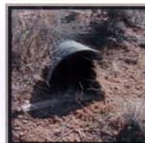
Burrow C Culvert Aspect: 355° (NE) Height: 23 cm Width: 35 cm
