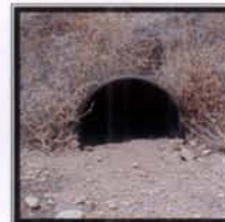
Burrow B Culvert Aspect: 130° (E) Height: 27 cm Width: 37 cm
