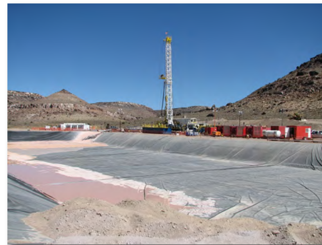
Lined Sump at ER-EC-11 to Hold Up to Four Million Gallons of Water During Well Drilling & Pumping Activities
