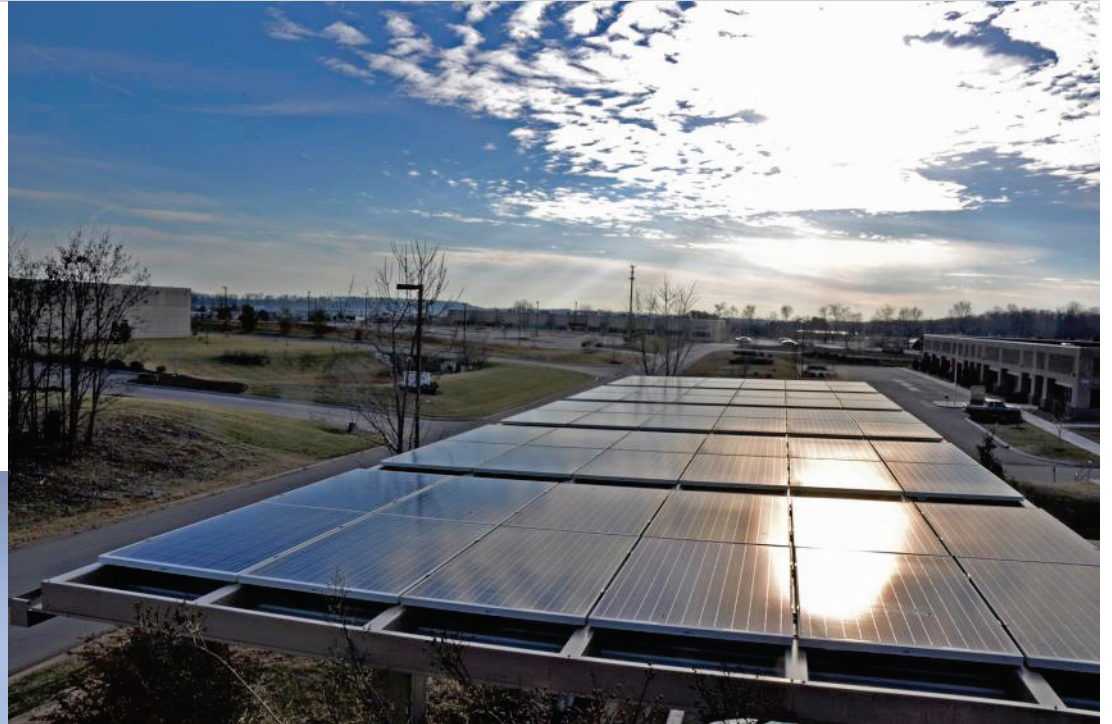
Roof-Top Solar Panels
