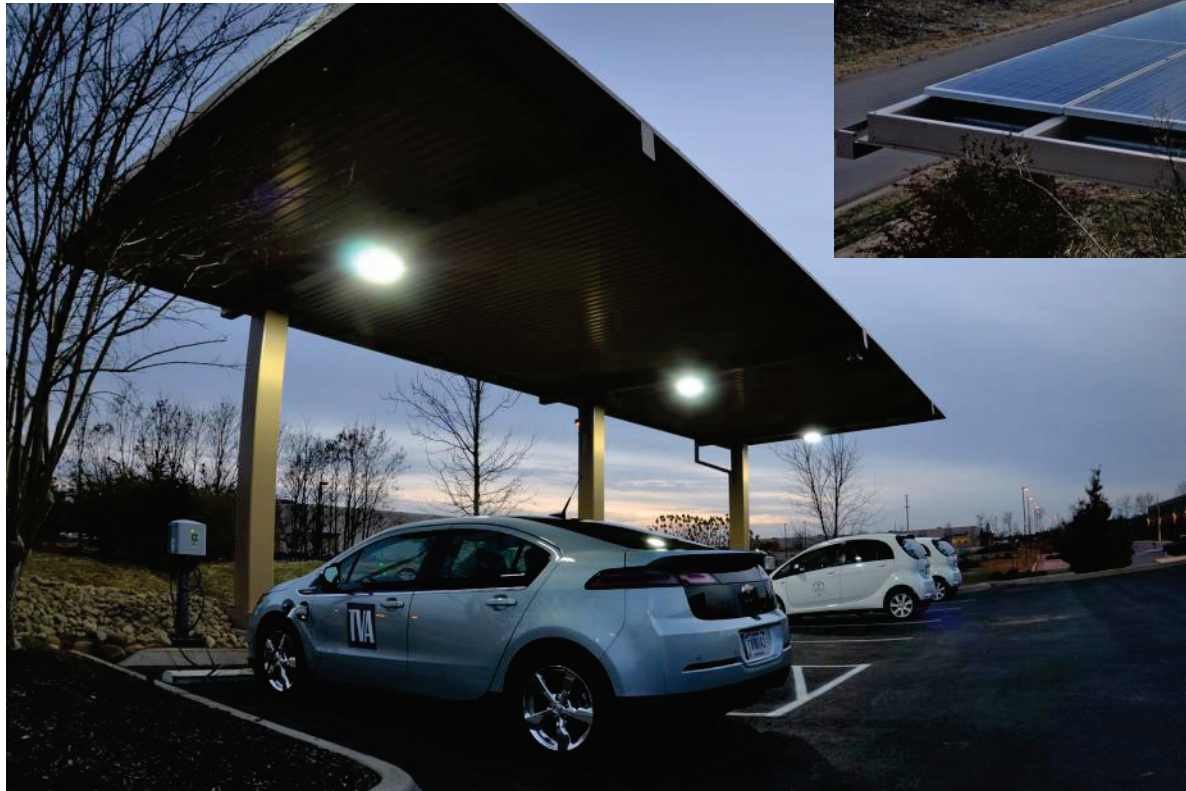
Electric Vehicles Charging
