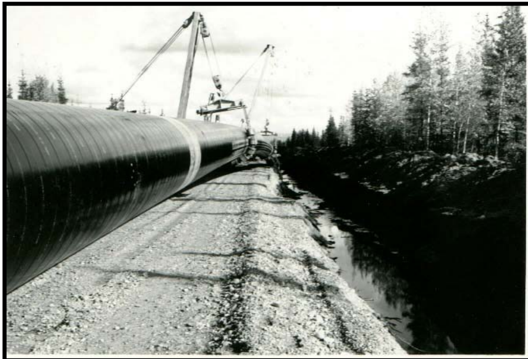
A portion of the Trans-Alaska pipeline that runs through Eielson AFB under construction
