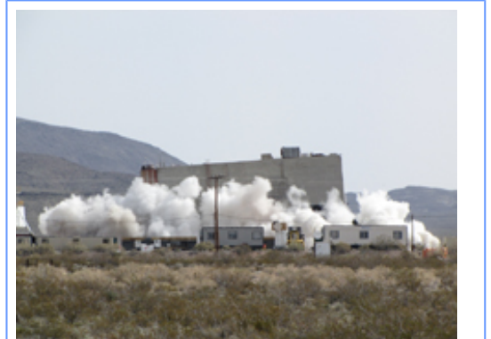
Crews perform demolition of the R-MAD facility. R-MAD is one of several Nevada Test Site facilities which supported the Nuclear Rocket Development Station program that ended in 1973.
