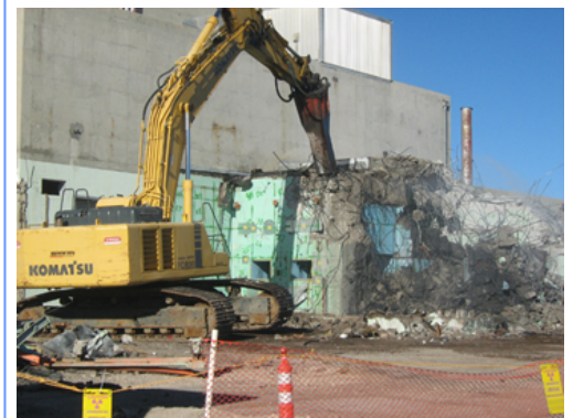
Phase I traditional demolition of R-MAD using a hydraulic hammer to dismantle a section of the south block wall and roof. A processor is used to size-reduce the resulting debris.
