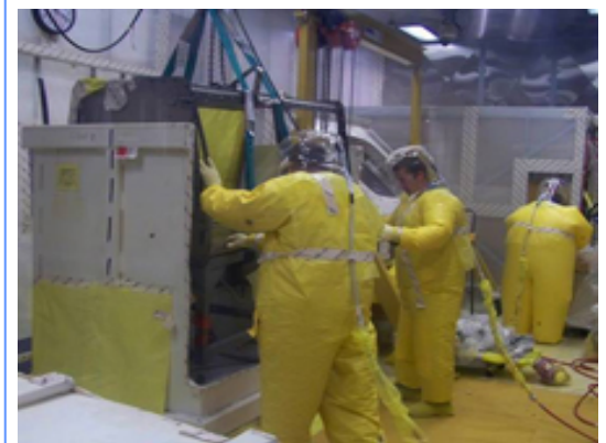
Workers in protective equipment remove a glovebox section after cutting open an oversized box.
