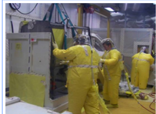
Workers in protective equipment remove a glovebox section after cutting open an oversized box.
