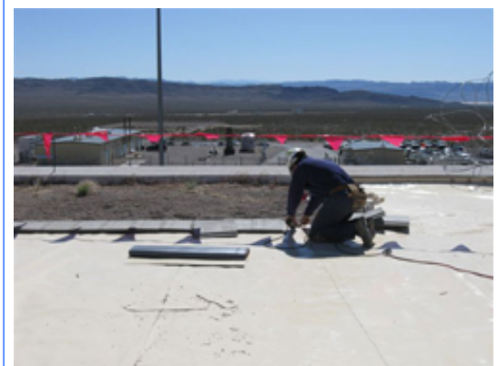
A worker places covering on the roof of the Device Assembly Facility (DAF).
