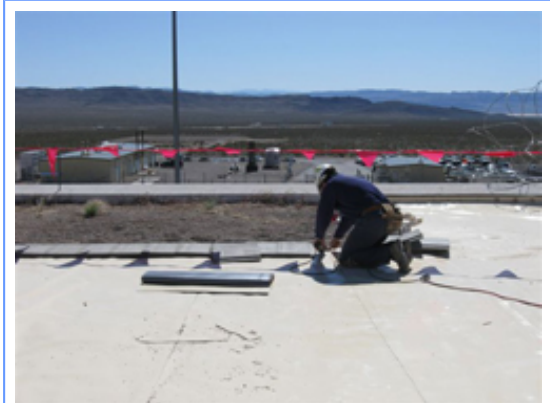
A worker places covering on the roof of the Device Assembly Facility.
