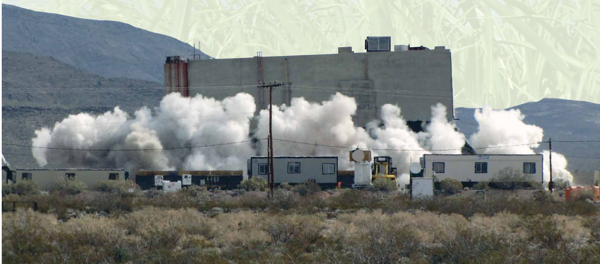
Controlled explosive demolition of R-MAD to safely bring the multi-story building down within reach of heavy equipment.
