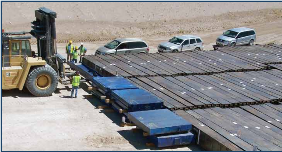
Steel shield doors from the demolition of R-MAD disposed as low-level radioactive waste at the NNSS Area 5 Radioactive Waste Management Site.
