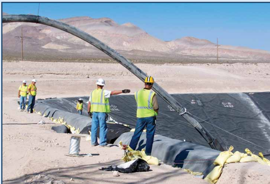
The U.S. DOE Environmental Management Program operates a RCRA-permitted Mixed Waste Disposal Unit at the Area 5 Radioactive Waste Management Site at the NNSS.
