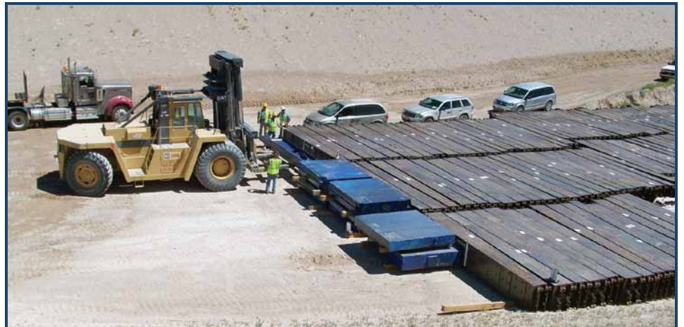
More than $54 million in accelerated environmental restoration activities have been completed at the NNSS, among them demolition and removal of debris from the Pluto Disassembly and Reactor Maintenance, Assembly and Disassembly (R-MAD) facility.
