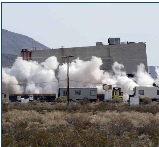
The NNSS used American Recovery and Reinvestment Act (ARRA) monies to clean up several outdated facilities at NNSS, among them the Reactor Maintenance, Assembly and Disassembly (R-MAD) facility.
