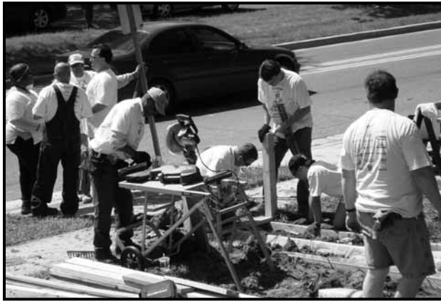
Members of the RSL-Andrews crew work to construct a wheelchair ramp for a homeowner in District Heights, Maryland.
