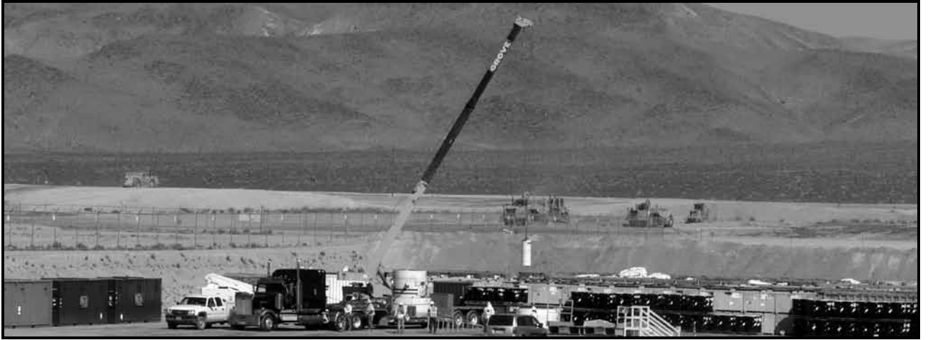
Waste Management personnel at NNSS have rigorous safety processes in place for disposing of low-level waste at Area 5 RWMS.
