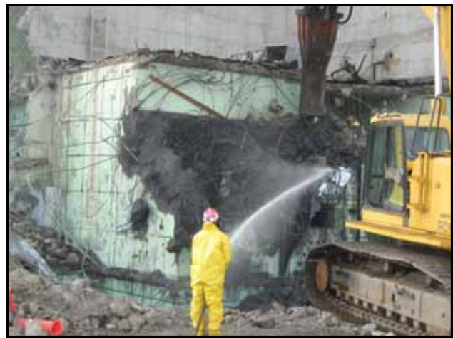
Crews perform demolition of the R-MAD facility. R-MAD is one of several NNSS facilities which supported the nuclear rocket program that ended in 1973.
